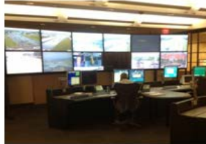
Central Computer System
