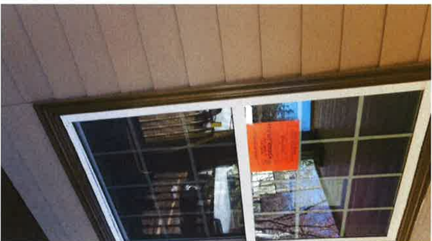
Close-up of installed windows – SDL, flush mounted, sills and original trim also removed
