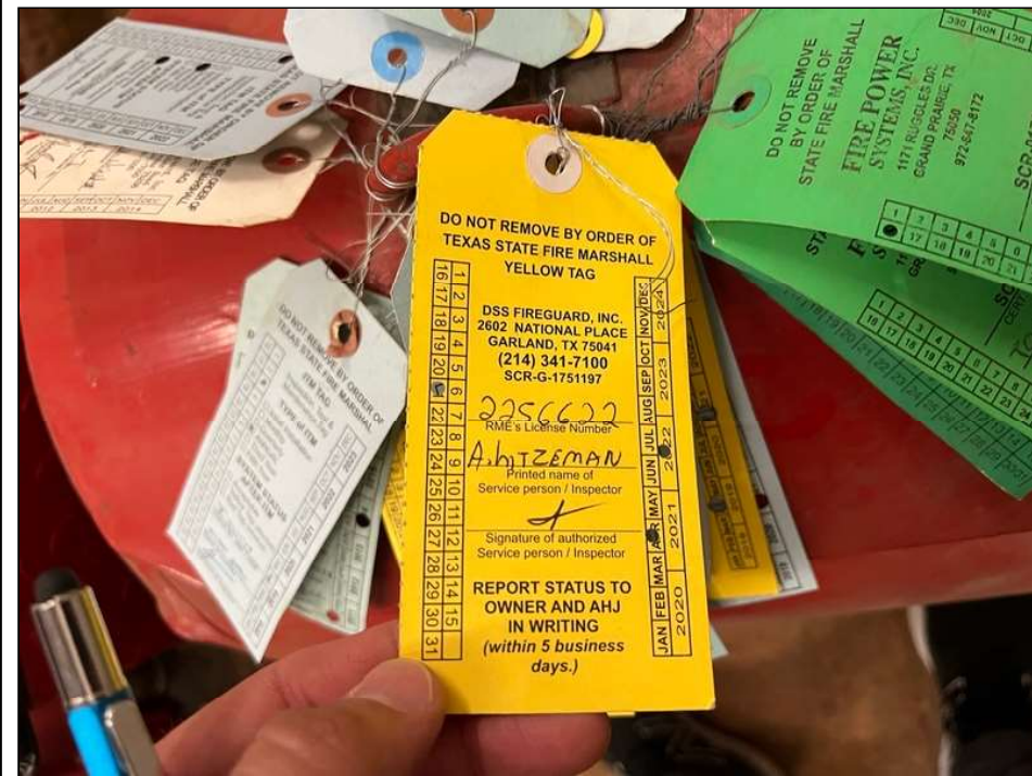
80. Yellow tags at fire sprinkler system
