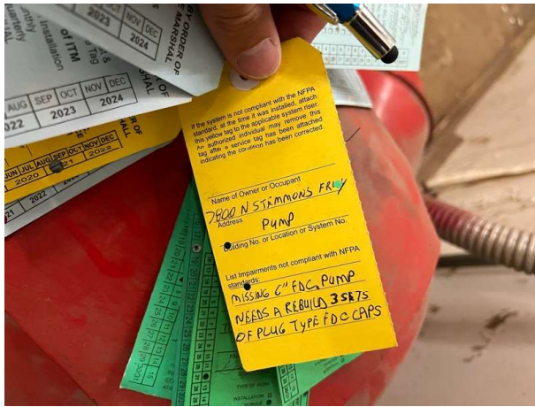
Yellow tags at fire sprinkler system
