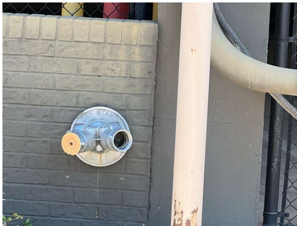
Missing FDC caps
