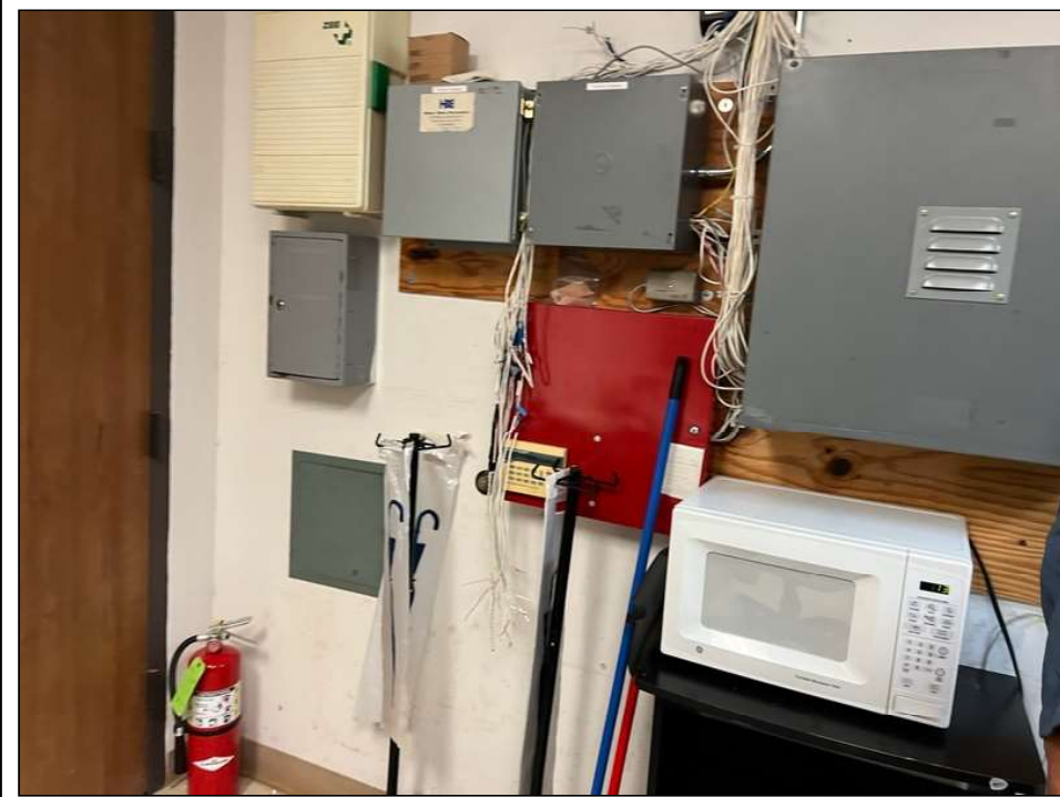
36. Fire alarm panels
