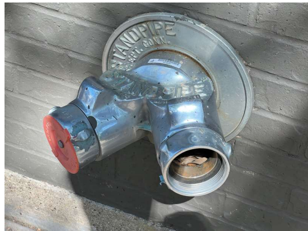
Missing FDC caps
