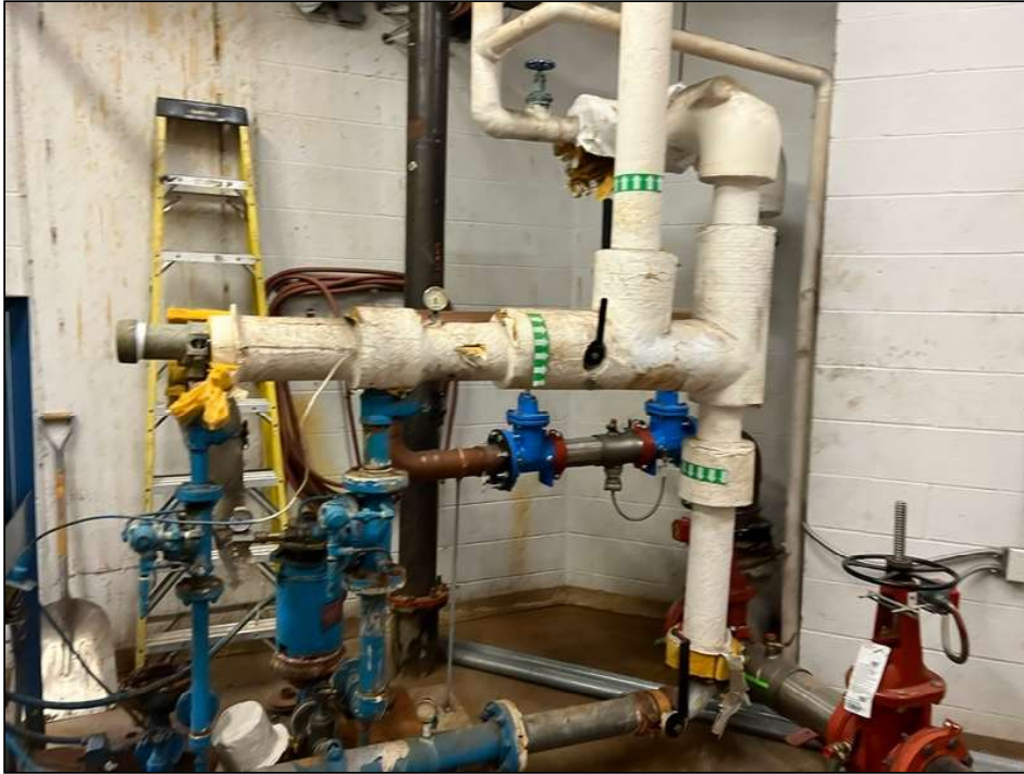
41. Chilled water piping
