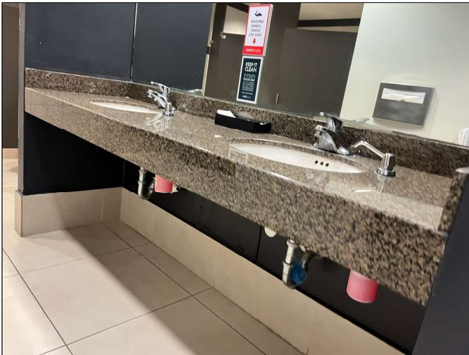
88. Sink pipe protection is needed
