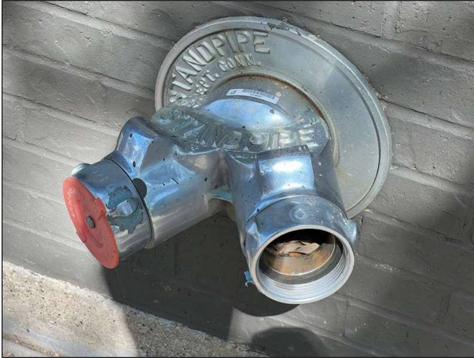
85. Missing FDC caps
