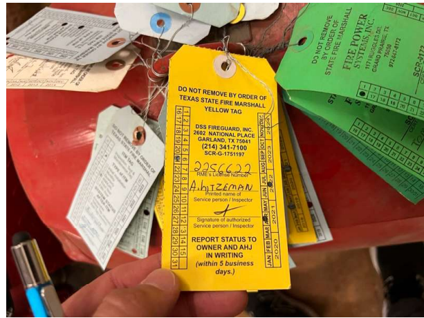
Yellow tags at fire sprinkler system
