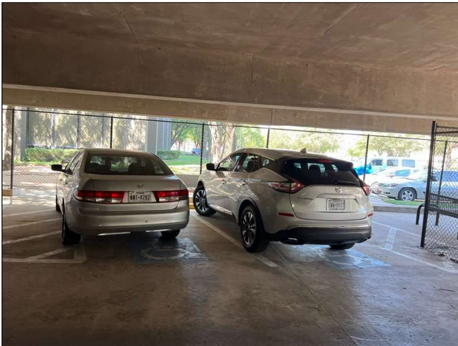
82. Missing accessible parking signs
