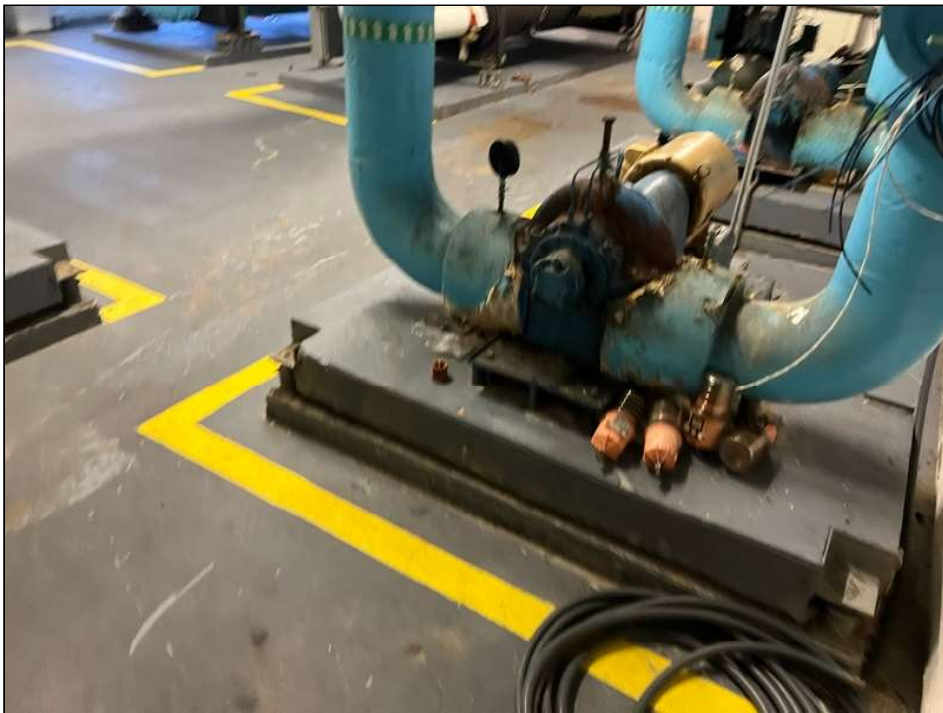
20. Domestic water pump
