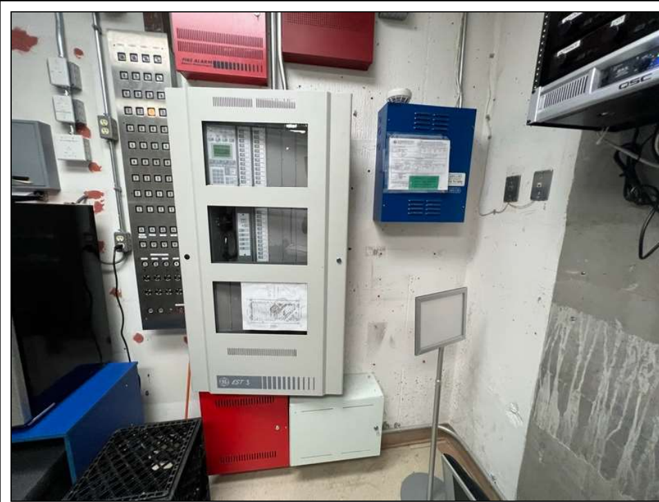
37. Fire alarm panel
