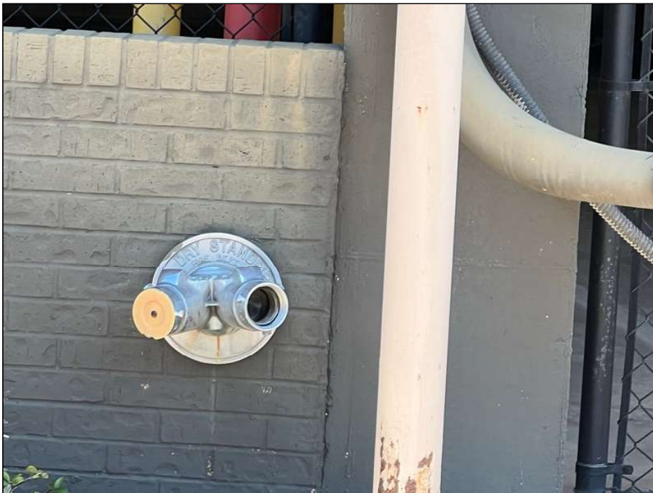
84. Missing FDC caps
