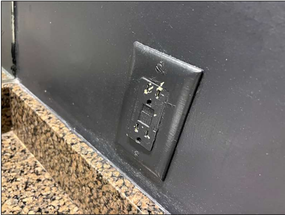
31. GFCI electrical outlet
