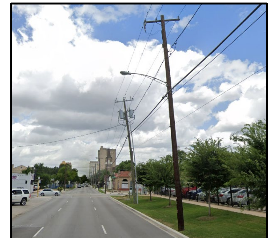
Example of lighting infrastructure in poor condition – leaning poles. (Haskell Ave. between Victor St. and Worth St).
