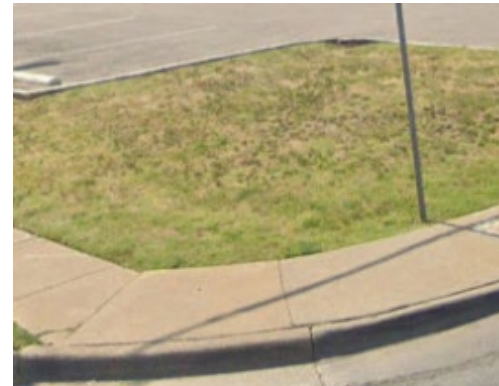
Curb ramps missing at American Way
