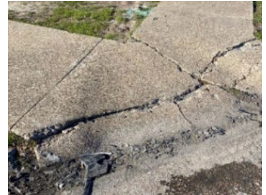
Ramps not ADA compliant
