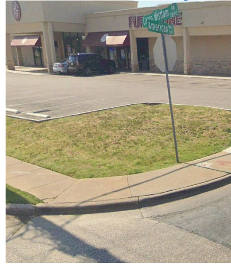
Curb ramps missing at American Way
