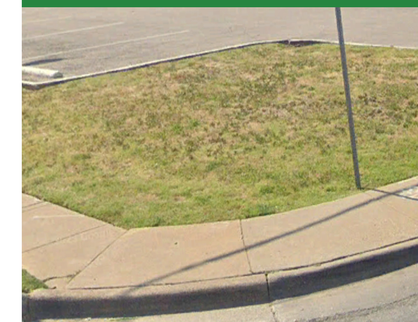
Curb ramps missing at American Way
