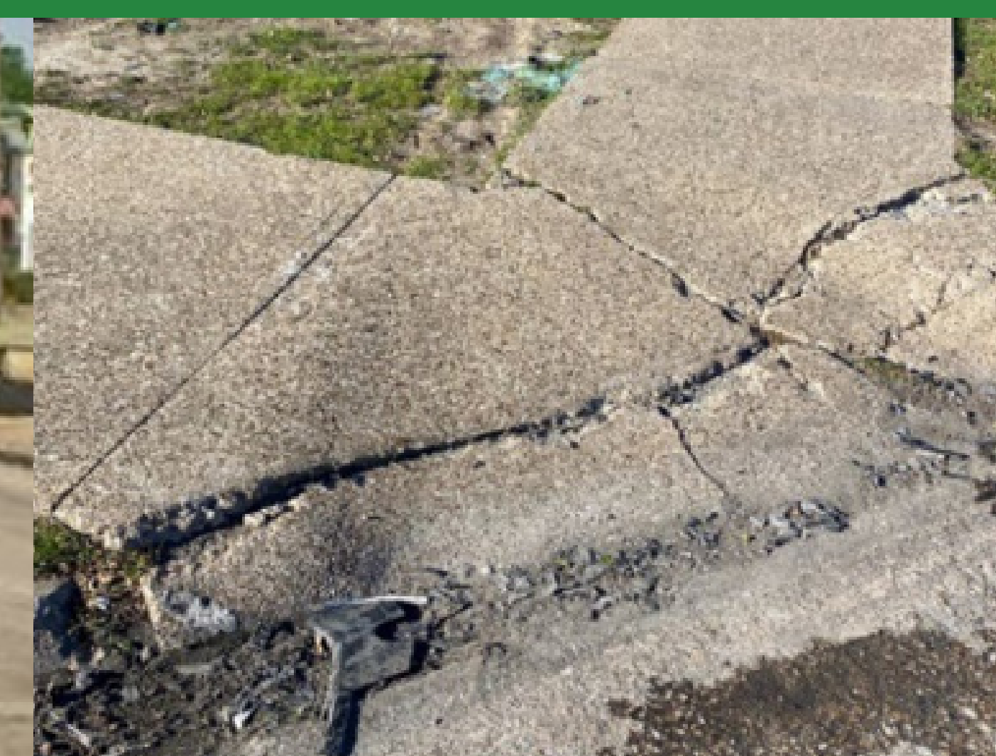
Ramps not ADA compliant
