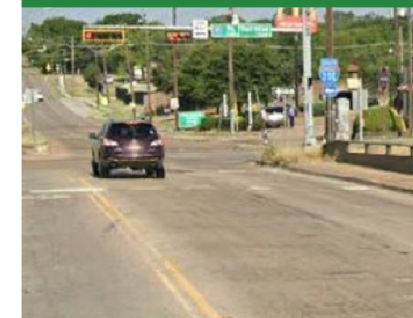
Faded pavement markings
