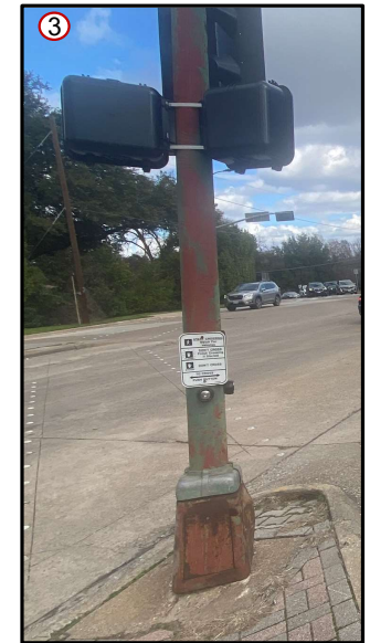
Pedestrian push buttons not up to ADA standards
