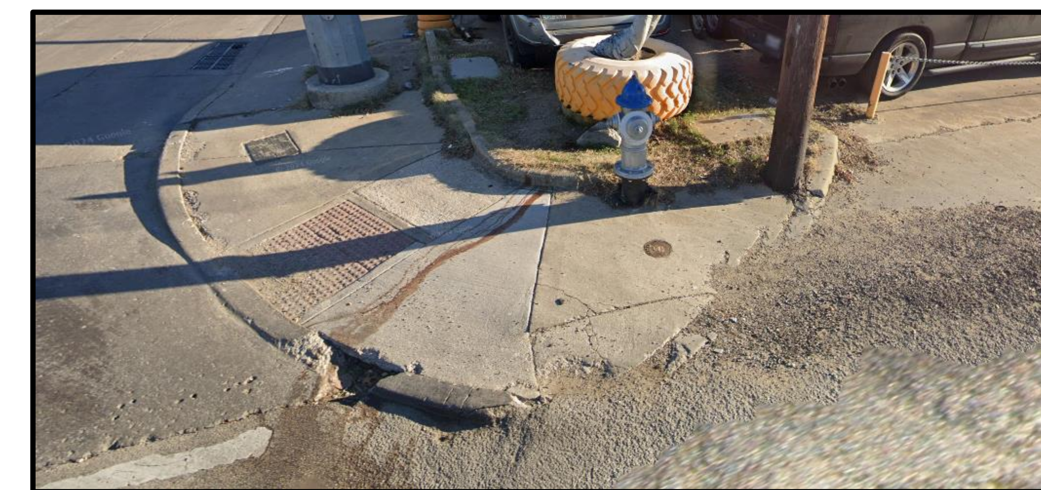
Example of a ramp in poor condition (South corner of Inwood & Maple). Several sections of the curb have broken off and the ramp is not ADA compliant.
