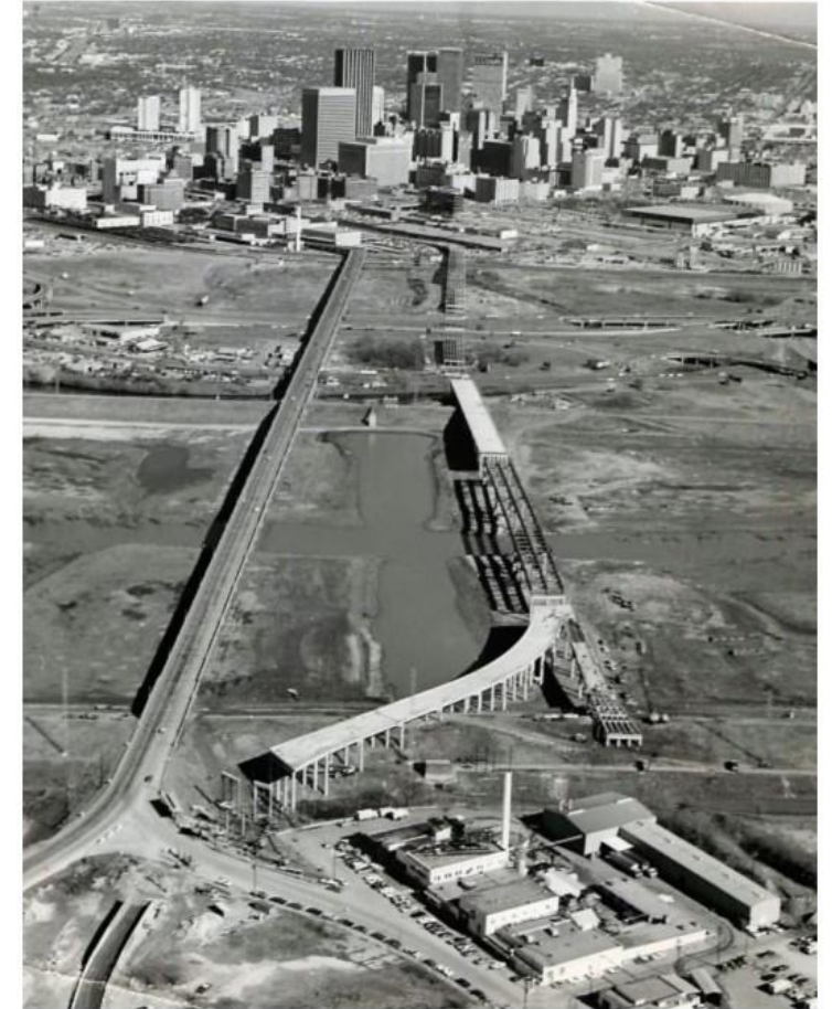
Jefferson Street Viaduct construction is shown on January 11, 1972. The Houston Street Viaduct is at left.
