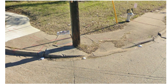
Ramps not ADA compliant
