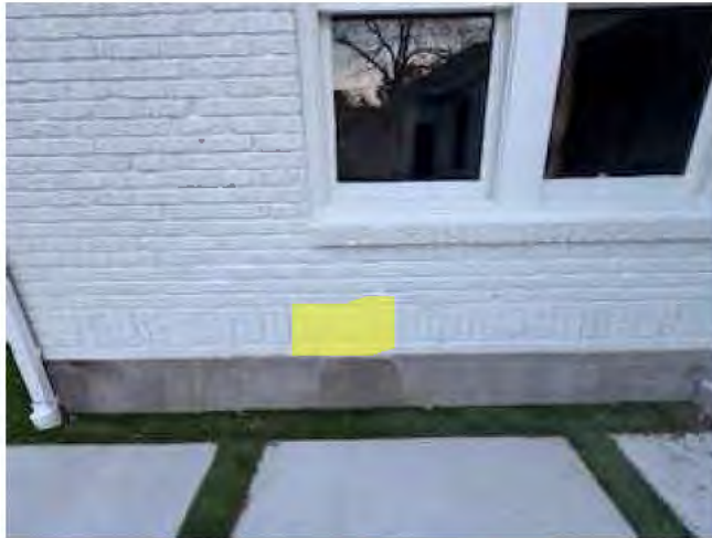
Back bedroom. We had to replace several cracked bricks in this area.
