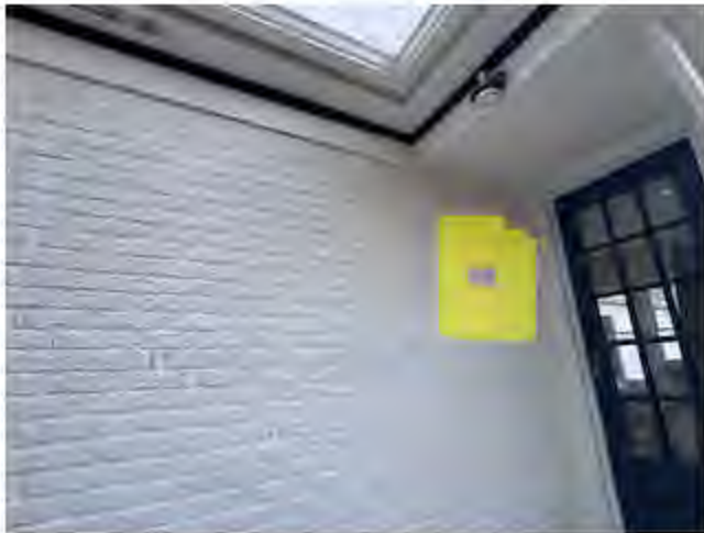
Back right bedroom entrance. We had to replace several cracked bricks in this area.
