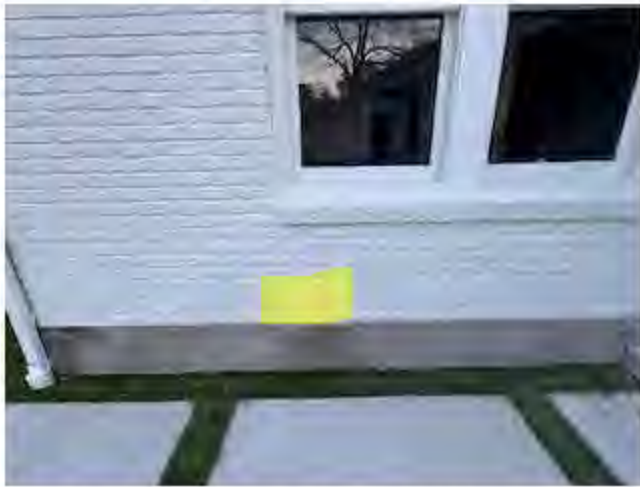
Back bedroom. We had to replace several cracked bricks in this area.
