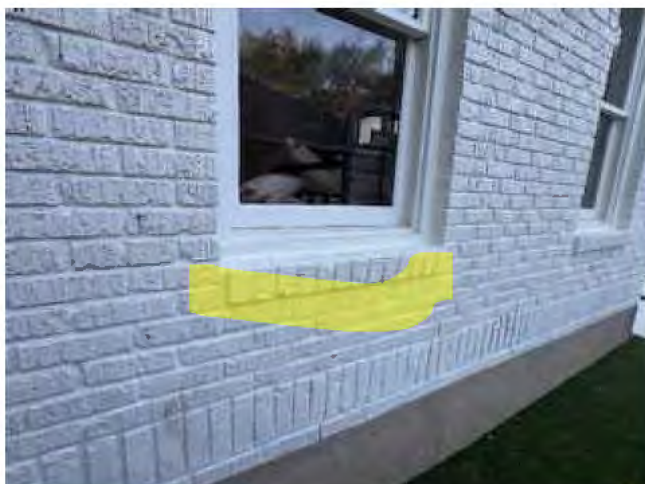
Back right bedroom window. We had to replace 4 to 5 cracked bricks in this area.
