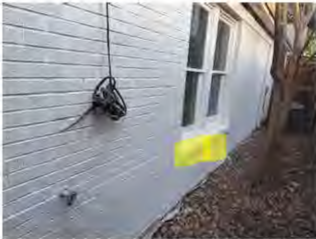
Back left window. We had to replace several cracked bricks in this area.
