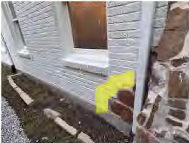
Front left-side window area. We had to replace several cracked bricks in this area.
