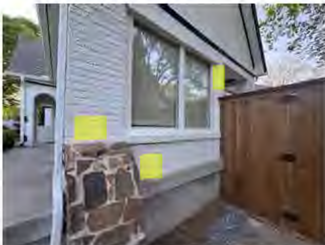
Front right-side area. We had to replace several cracked bricks in this area.
