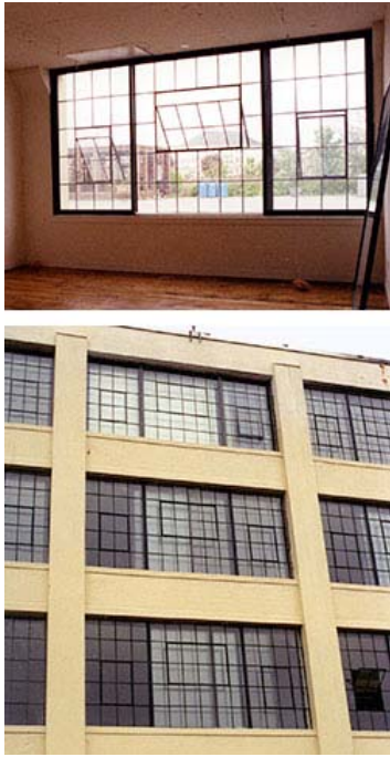
Figure 15. Original steel windows were retained and made operable during the rehabilitation of this historic mill complex. Insulated sliding windows were added on the interior to improve energy efficiency.
