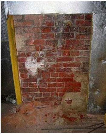
Figure 21. The interior face of a brick masonry wall shows damage that resulted from the installation of a vapor retardant (foil facing) and thermal insulation. Photo: Simpson Gumpertz & Heger.
