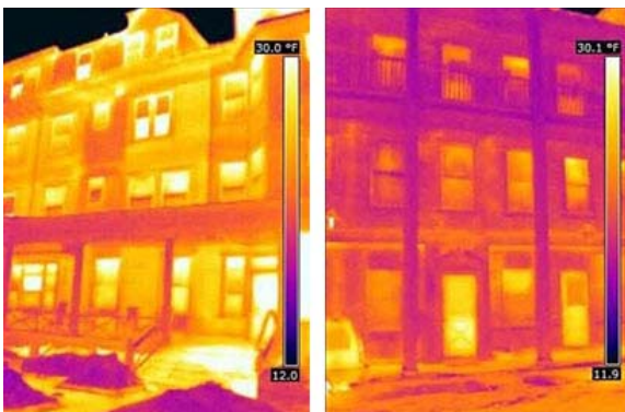
Figure 7. The left thermal image shows the walls of this building before insulating. After insulation was added, the cooler and, thus darker exterior walls evidence how much the heat loss has been reduced. Photos: EYP Architecture & Engineering.
