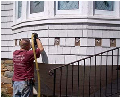
Figure 18. Dense-packed cellulose insulation is being blown in through holes drilled in the sheathing. Once the operation has been completed, the shingles will be reinstalled. Photo: Edward Minch.
