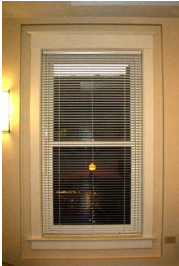
Figure 20. The walls have been furred out inappropriately around the historic window trim creating an appearance the interior never had historically.
