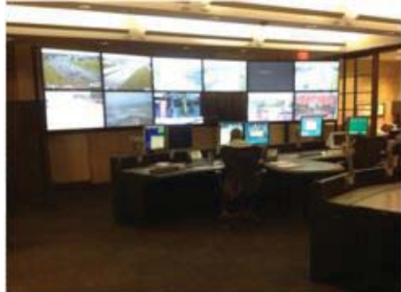
Central Computer System
