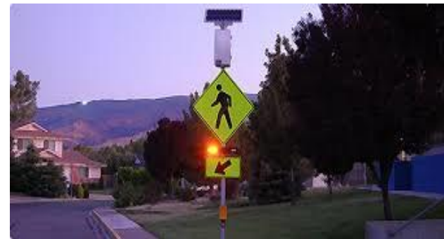
Rectangular Rapid Flashing Beacons
