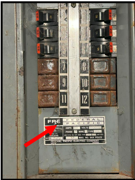
Obsolete electrical subpanel
