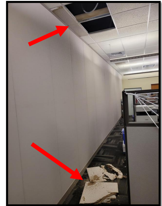
Collapsed ceiling in L1 Payroll due to water infiltration
