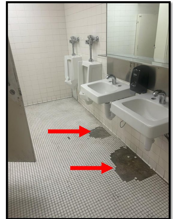
Restroom facilities beyond serviceable life
