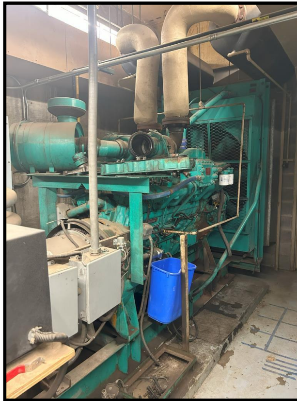
Non-functional and obsolete emergency generator
