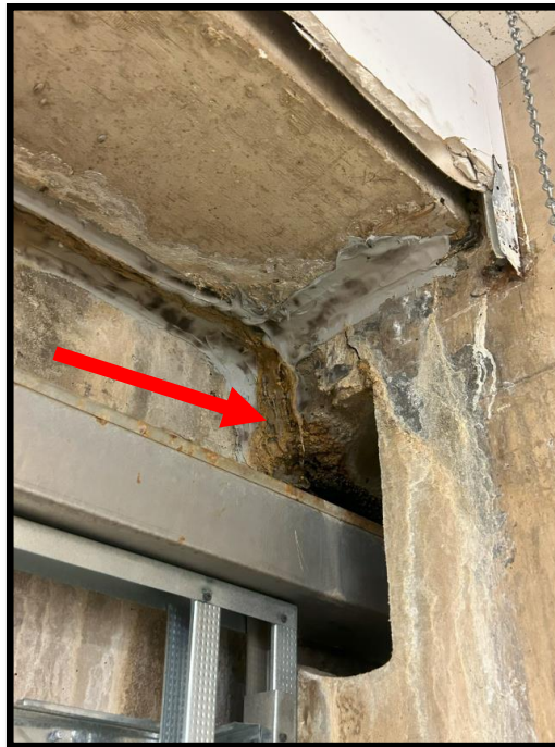
Failed interior gutter system
