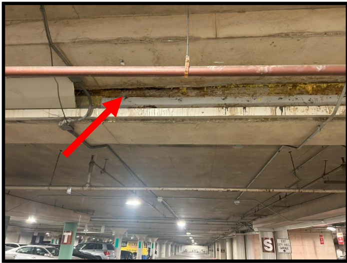
L1 garage structural and water infiltration
