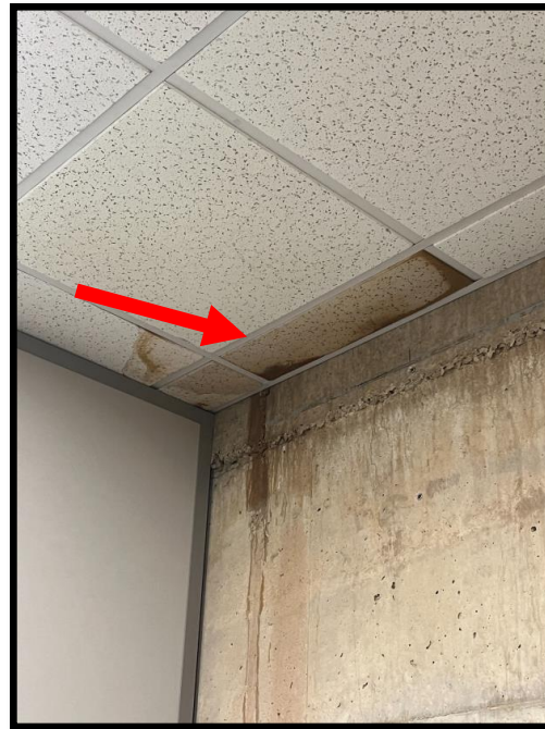
Water infiltration in L1 Payroll offices
