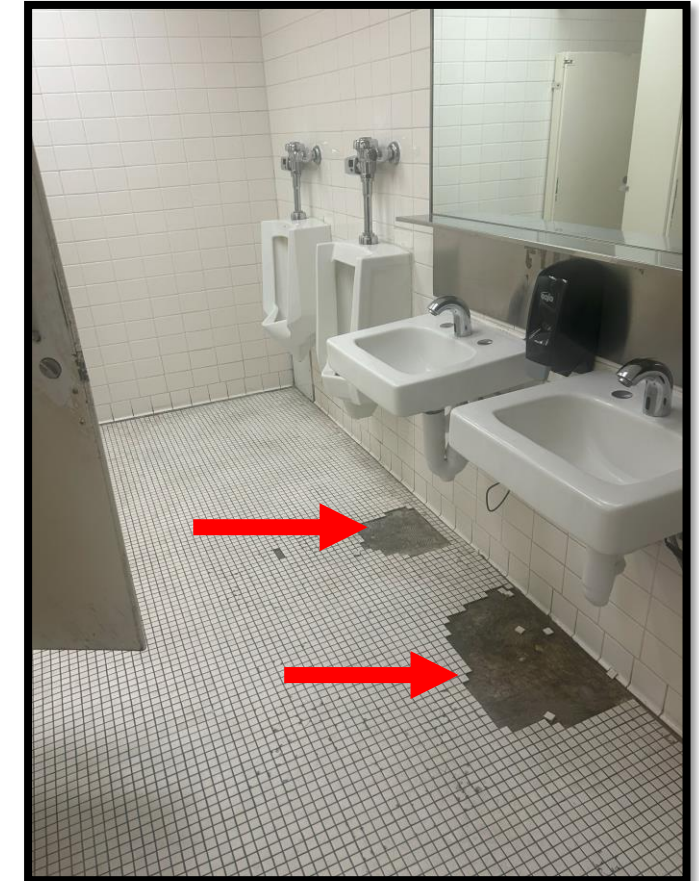
Restroom facilities beyond serviceable life
