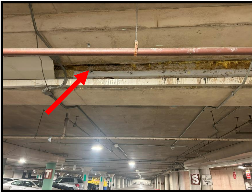
L1 garage structural and water infiltration
