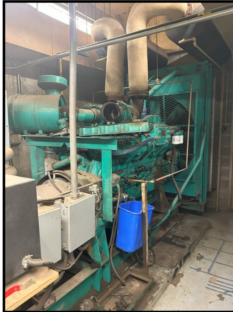
Non-functional and obsolete emergency generator
