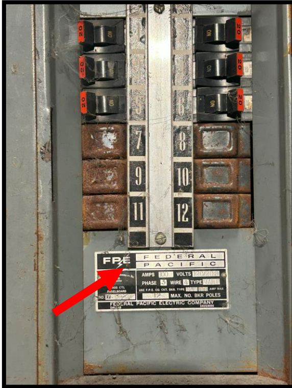
Obsolete electrical subpanel
