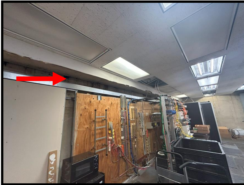
Active water infiltration over a telecommunications distribution center w/failed gutter system
