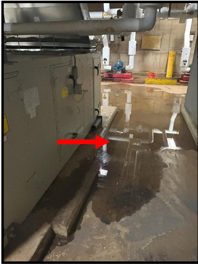
8 th floor water infiltration
