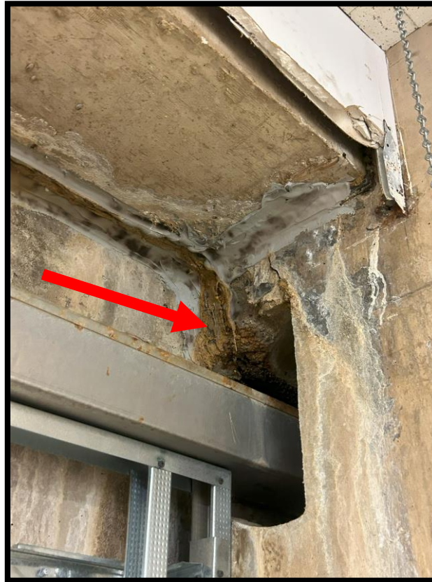
Failed interior gutter system
