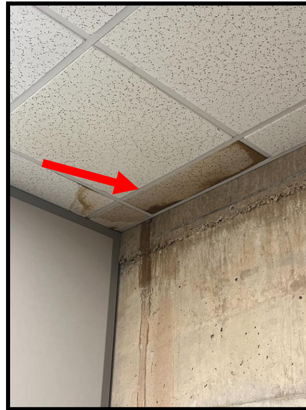
Water infiltration in L1 Payroll offices
