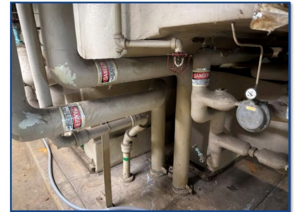
HA 58: 4" TSI Pipe Insulation Runs (Tan)
