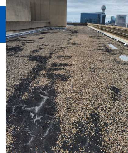
Typical condition of roof membrane, exhibiting widespread surface deterioration and nearing end of typical service life.
