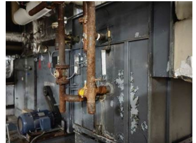
Original HVAC Equipment with Corroded Piping
