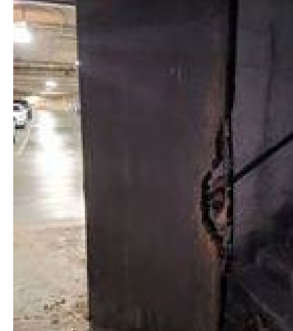
Corroded interior door of parking garage interior stairwell
