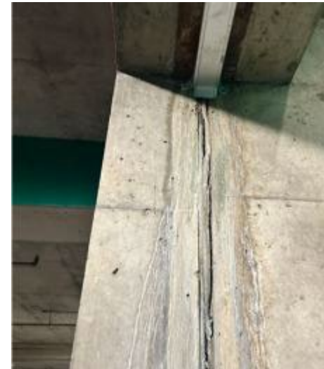
Cracking and distress at expansion joints, signs of water intrusion.
