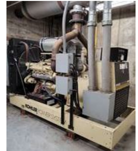
Aged emergency generators; multiple units beyond typical service life
