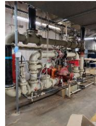
Fire suppression wet system
