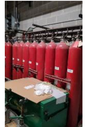
Aged clean agent fire suppression system
