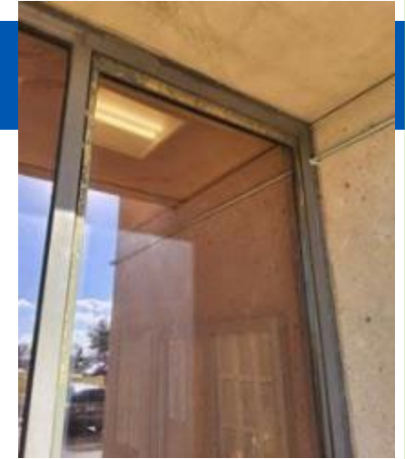
Original aluminum-framed windows do not meet current energy code requirements
