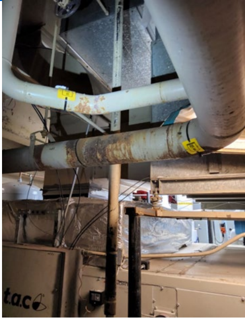
Corrosion on Mechanical Piping
