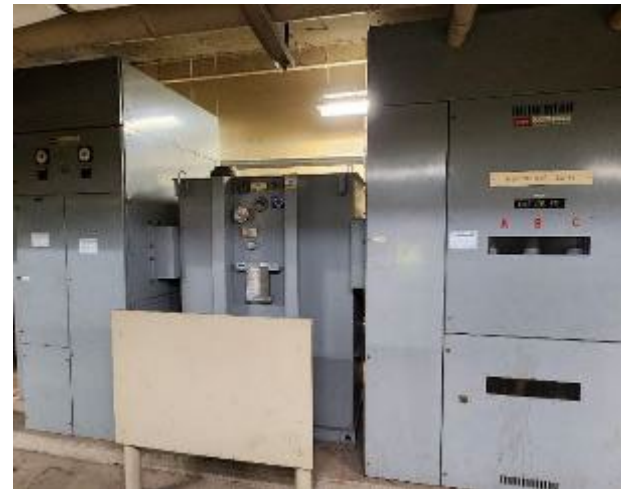
Original switchgear has exceeded typical service life
