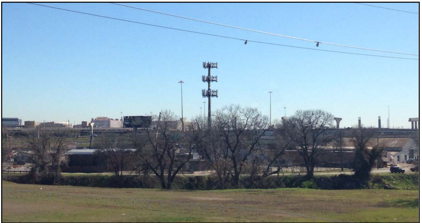
Extended 95' Monopole Tower
