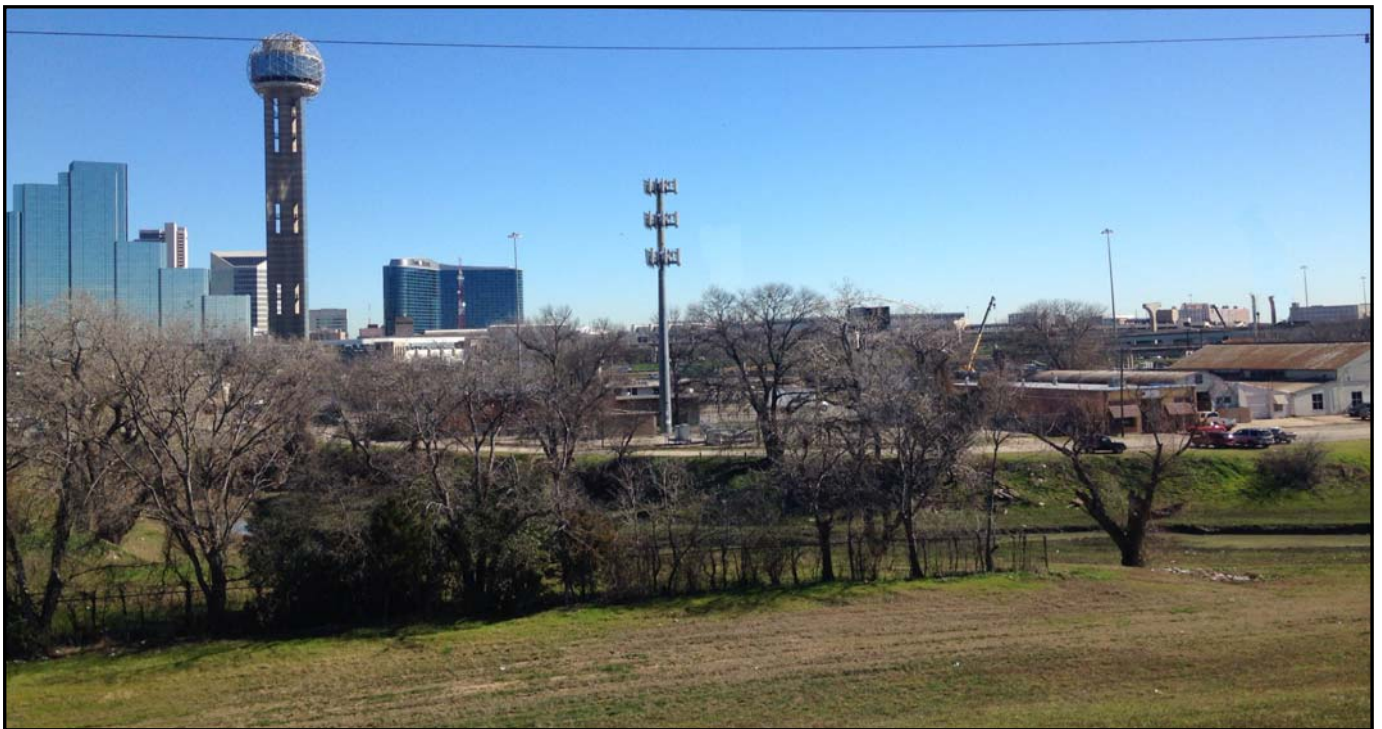
Extended 95' Monopole Tower
