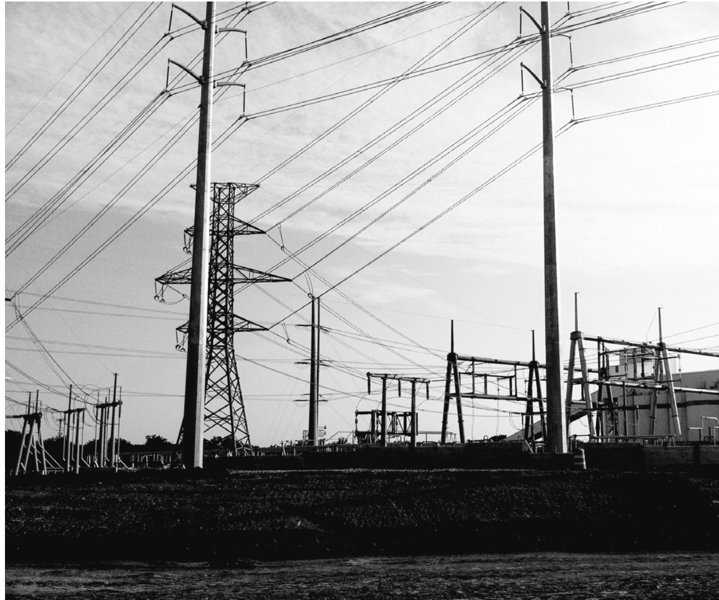
Oncor West Levee Substation
