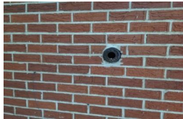
Missing Wall Clean-out Plug
