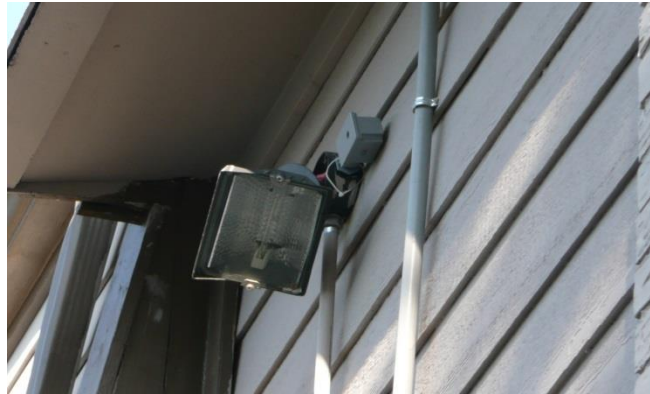
Violation – security light not in working order.
