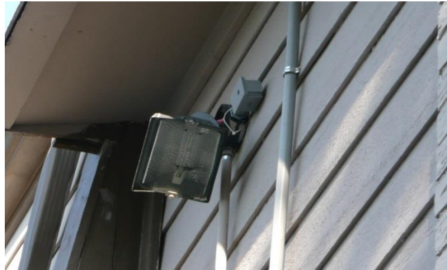
Violation – security light not in working order.
