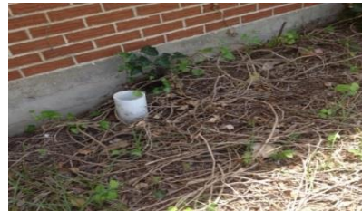
Missing Clean-out cap
