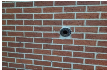
Missing Wall Clean-out Plug
