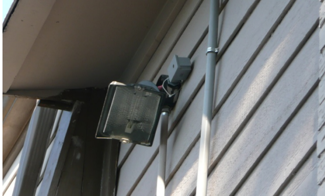
Violation – security light not in working order.
