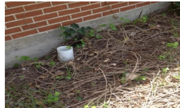
Missing Clean-out cap
