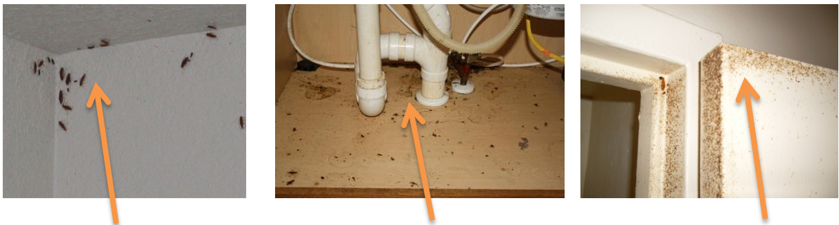
Infestation of roaches on walls and under kitchen sinks. Excretion of roaches
