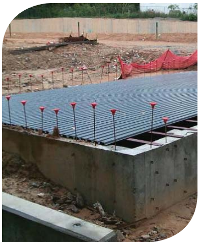
Detention storage located in underground pipe and tank systems.
