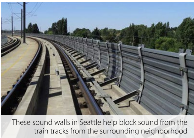
Sound walls can be built into tracks in an aesthetically appealing way while also minimizing sound impacts
