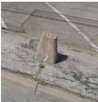
ABOUT A DOZEN UTILITY STUMPS EXIST THROUGHOUT THE MEDIANS CURRENTLY.
