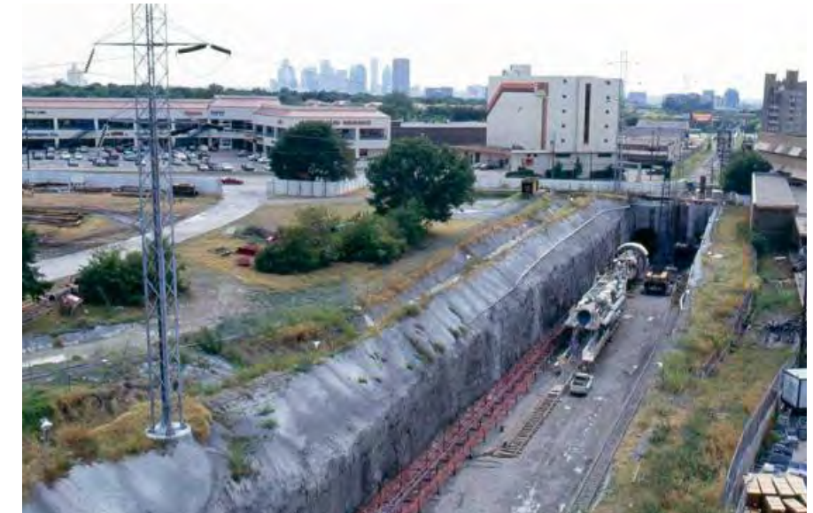
The DART train portal constructed as part of the D2 project should be minimally intrusive and allow for air rights development. Source: DART
