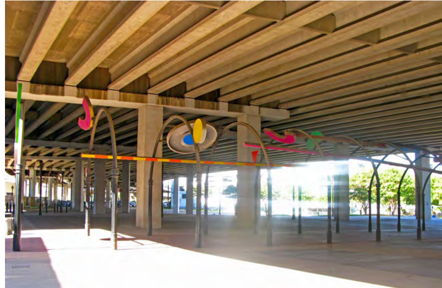
A safer, better lit connection under Woodall Rodgers Freeway will create a stronger connection between Victory Park and the West End.
