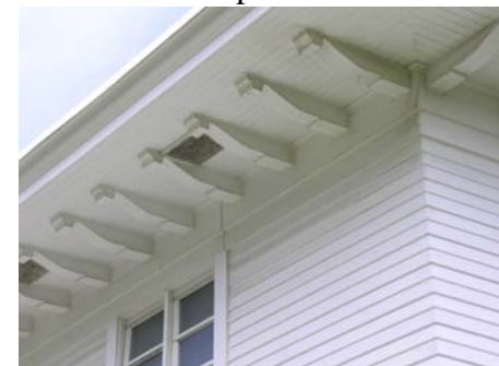
Screened eave vent
