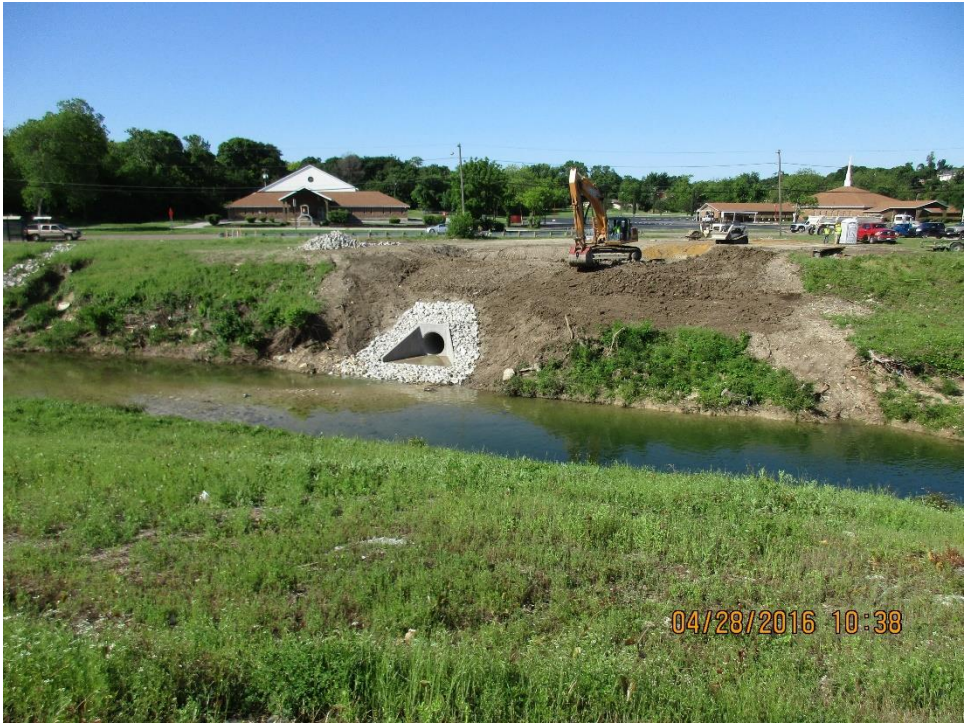
Ledbetter Storm Drainage Project Upsizing a failed 48" Metal Pipe to 60" Reinforced Concrete Pipe (2016)
