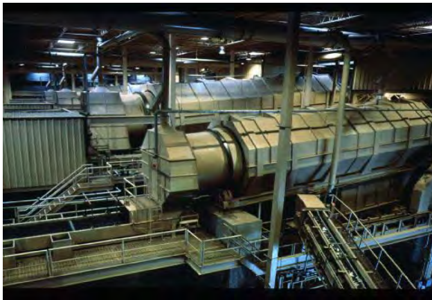
Figure 3 - RDF Processing Facility, Virginia
