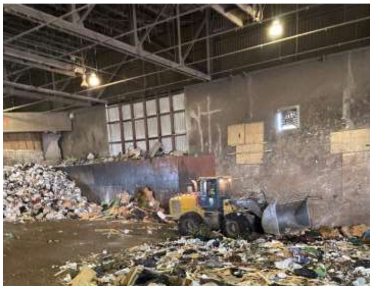
Figure C-7: Waste Storage Pit Wall Structural Damage at Bachman Facility
