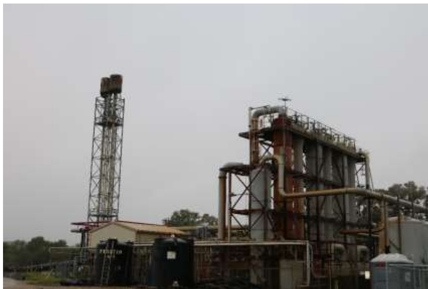
Figure E-19: Landfill Gas-to-Energy Plant
