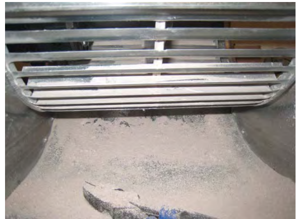
FP 15-15: Inside View of VAV Box Housing
