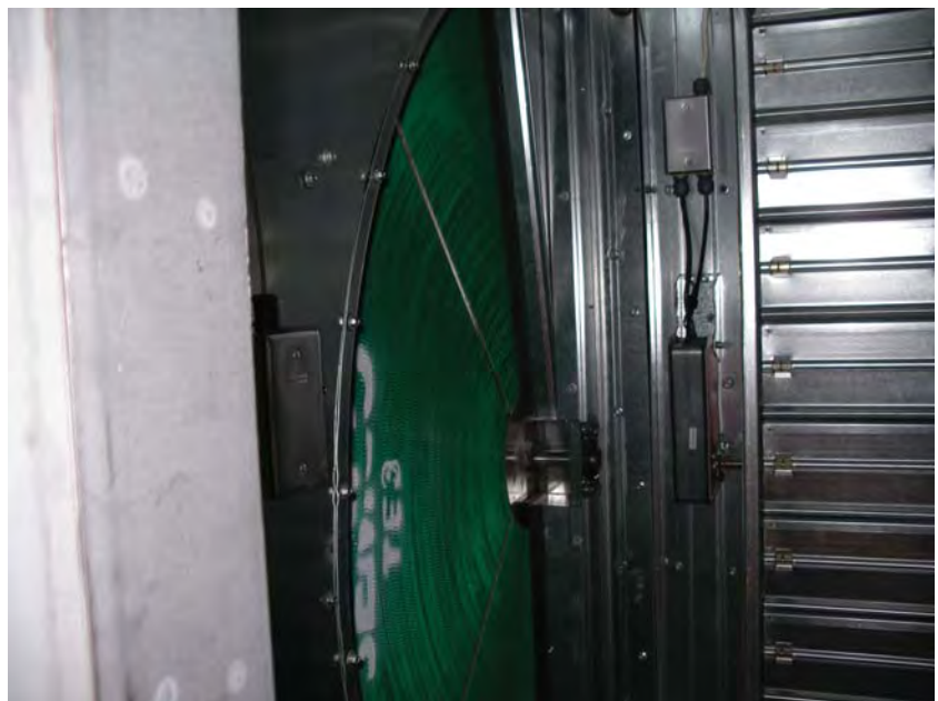
An Enthalpy Wheel Will help to Counteract Increases in Energy Consumption. Image provided by the Sidwell Friends School.
