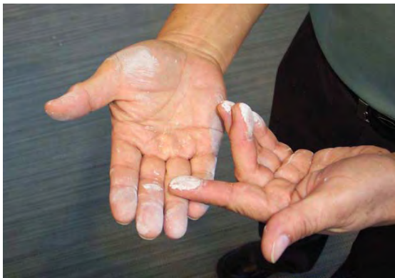
Drywall Dust Removed from the Face of Airflow Ring in the VAV Box.
