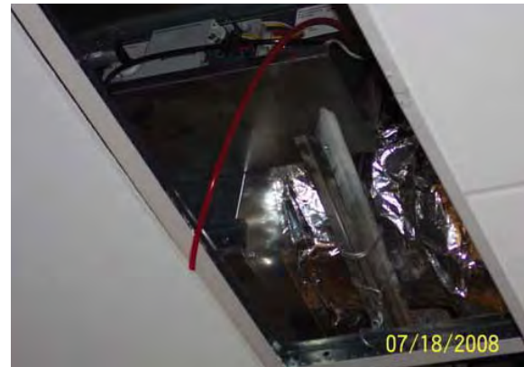
Metal Housing on Honeywell Controls is Missing.
