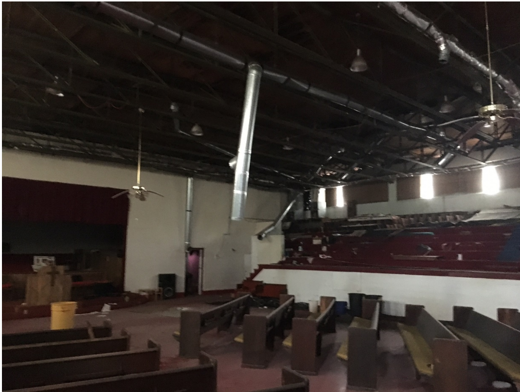
Gym/auditorium interior with an open truss ceiling, built-in bleachers, and a stage area for performances.
