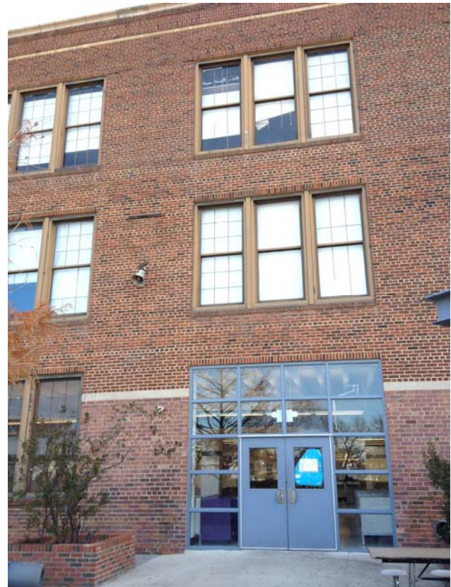
Original windows have been removed and new exterior doors and storefront installed in their place at west facade
