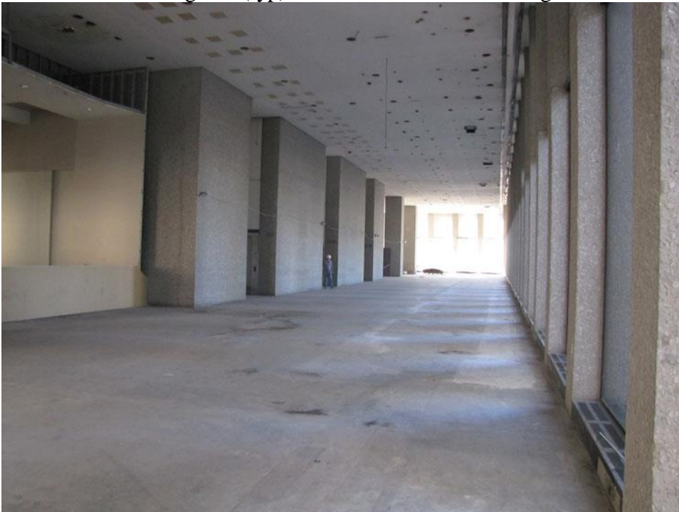
TX_Dallas County_One Main Place_0016 Second floor banking hall (typ) – south side – camera facing east
