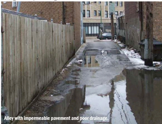
Figure P6. The Chicago Green Alley program uses porous paving to help manage stormwater runoff
