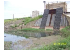
Pavaho (drainage area - 1,843 acres) 7 pumps – 666,720,000 GPD
