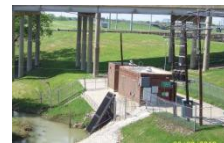
Charlie (drainage area - 779 acres) 3 pumps – 123,840,000 GPD
