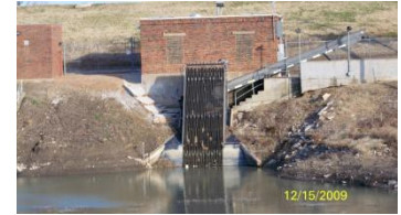
Delta (drainage area - 815 acres) 3 pumps – 129,600,000 GPD
