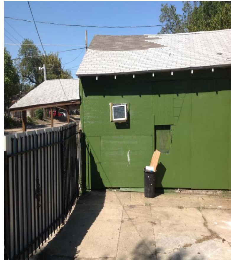
Illegal Outside Storage, Litter and Substandard Structure Abated
