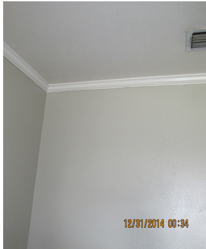
Interior Walls Painted after Bed Bug Extermination
