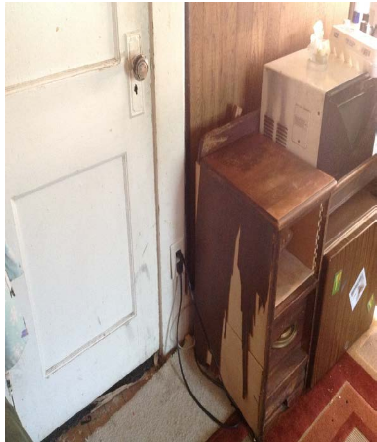
Electrical Violation Abated
