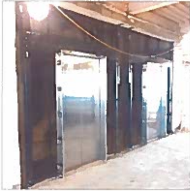
Elevator openings were cleared and new frames, sills and doors are installed on 15 floors
