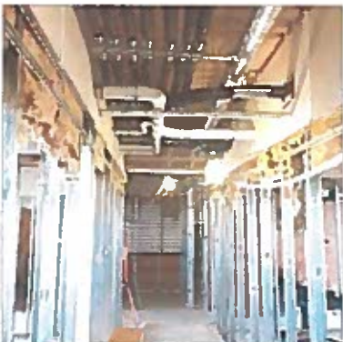
Dry wall, insulation, and fire tape at ceiling is completed on 17 apartment floors
