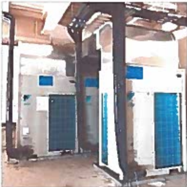
28 high energy efficient VRV HVAC units are installed
