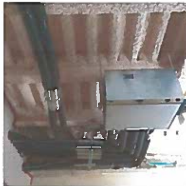
New fireproofing and fire safing (not pictured) is completed throughout the tower
