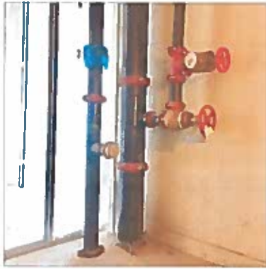
Four (4) fire sprinkler standpipes are installed (standpipe pictured in west-end staircase)
