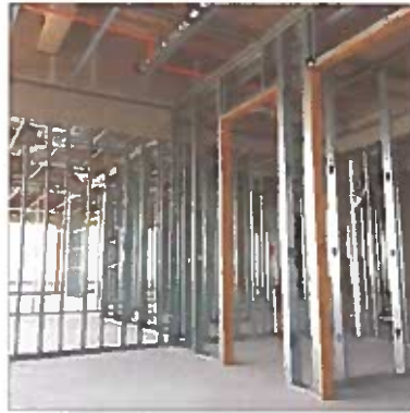
89% of steel unit separation wall framing is completed on 32 floors; 309 apartments and 174 hotel rooms have wall framing
