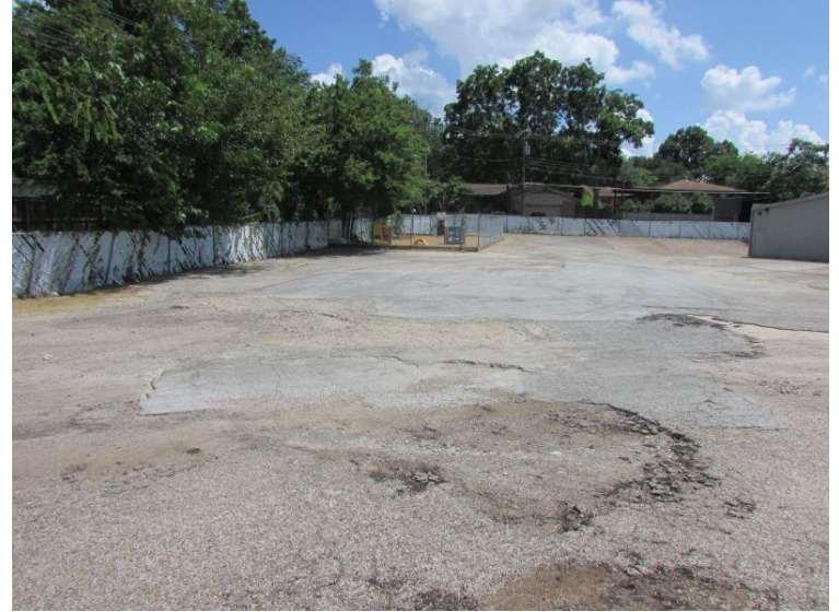
Deteriorated site conditions
