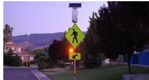
Rectangular Rapid Flashing Beacons
