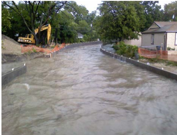
Elam Creek Phase I Providing 100-yr storm protection Before and during construction (2008)
