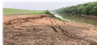
Erosion on Trinity River
