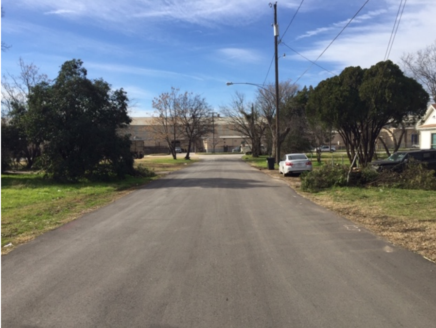
“A” Condition - New street that rides well with little to no cracks.
