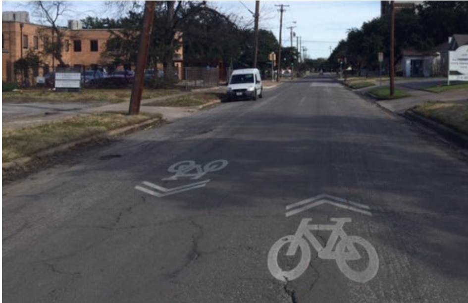
“C” Condition - Weather and Structural cracking becomes more prominent, rutting has started to develop.
