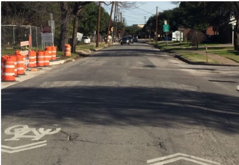
“D” Condition - Weather and structural cracking begins to widen and expand over 50% of the street, rutting is more pronounced raveling has begun.
