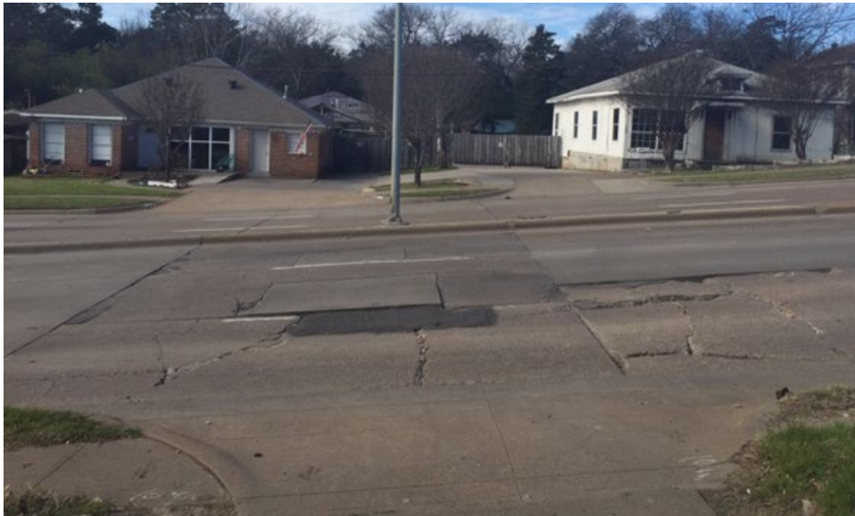
“E” Condition – Structural cracking covers over 50% of the street and frequent potholes are present.
