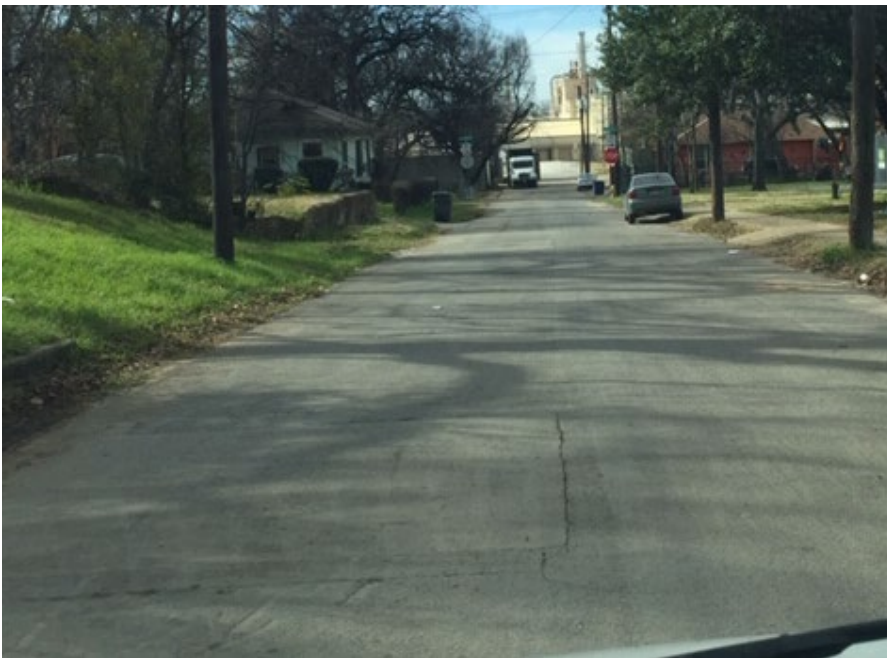
“B” Condition – Street has aged, ride is still smooth, but temperature cracks or utility cuts have been made.
