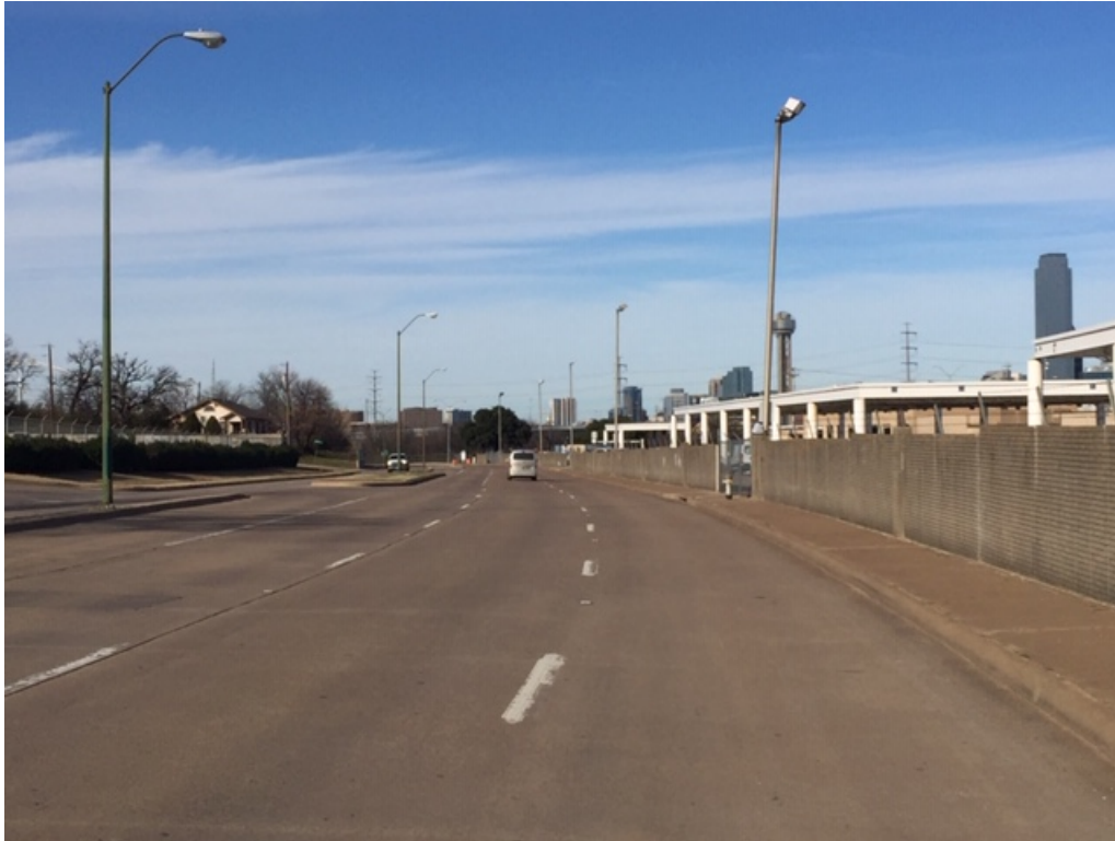
“B” Condition – Street has aged, ride is still smooth, but temperature cracks or utility cuts may have been made.
