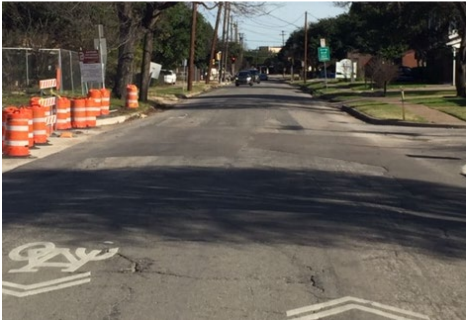
“D” Condition - Weather and structural cracking begins to widen and expand over 50% of the street, rutting is more pronounced raveling has begun.
