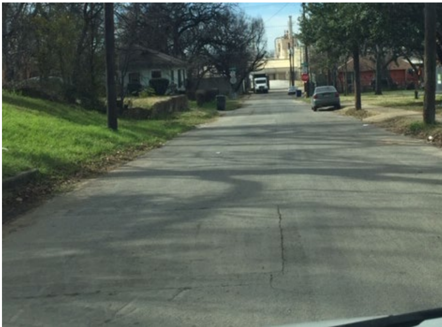
“B” Condition – Street has aged, ride is still smooth, but temperature cracks or utility cuts have been made.
