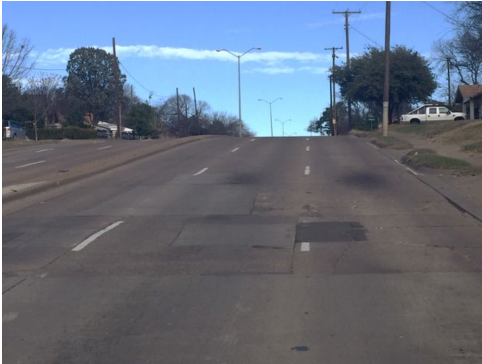
“D” Condition - Weather and structural cracking begins to widen and expand up to 50% of the panels.
