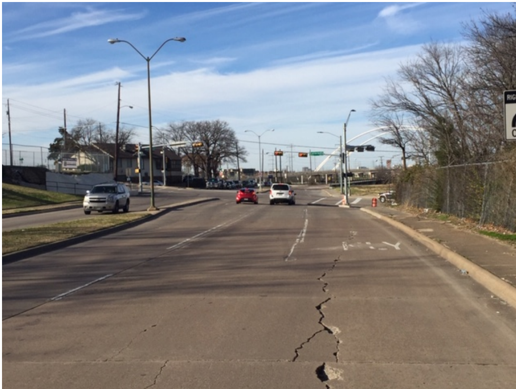
“C” Condition - Weather and Structural cracking becomes more prominent.
