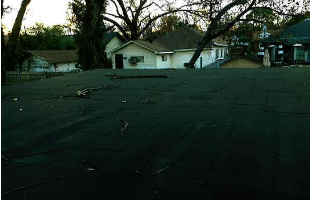
Rear porch flat roof. Photo submitted by applicant.
