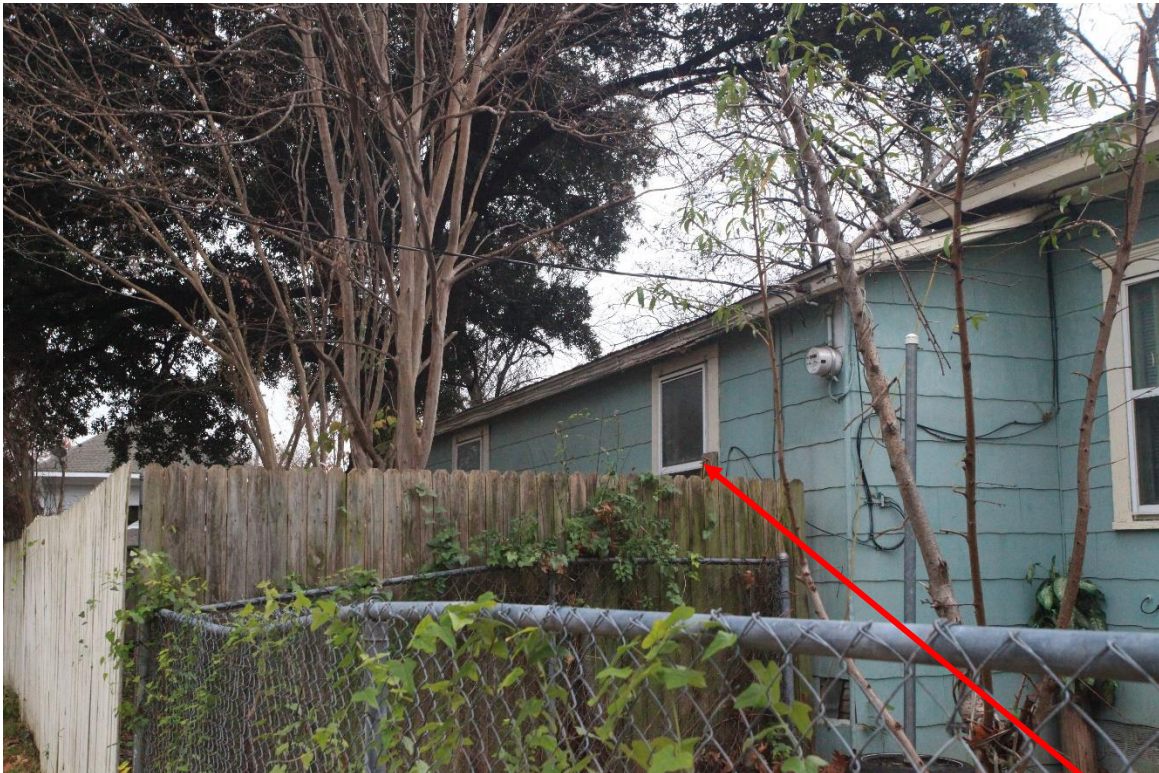
Request #2 – Close up view of left (East) side elevation with window proposed for resizing and relocation.
