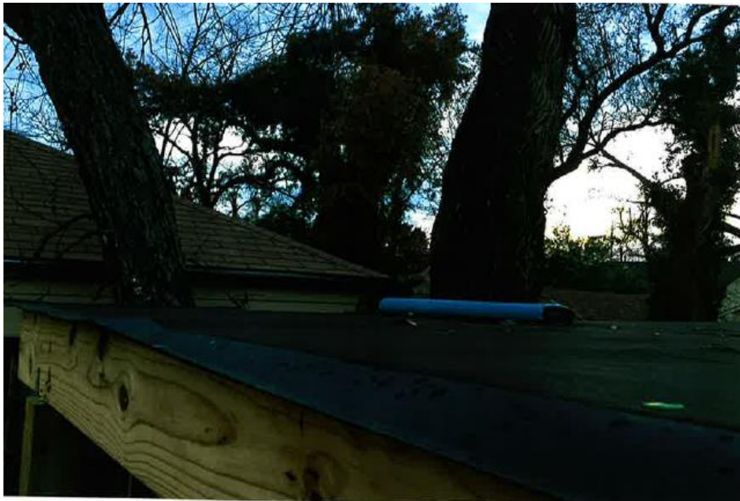
Rear porch flat roof. Photo submitted by applicant.
