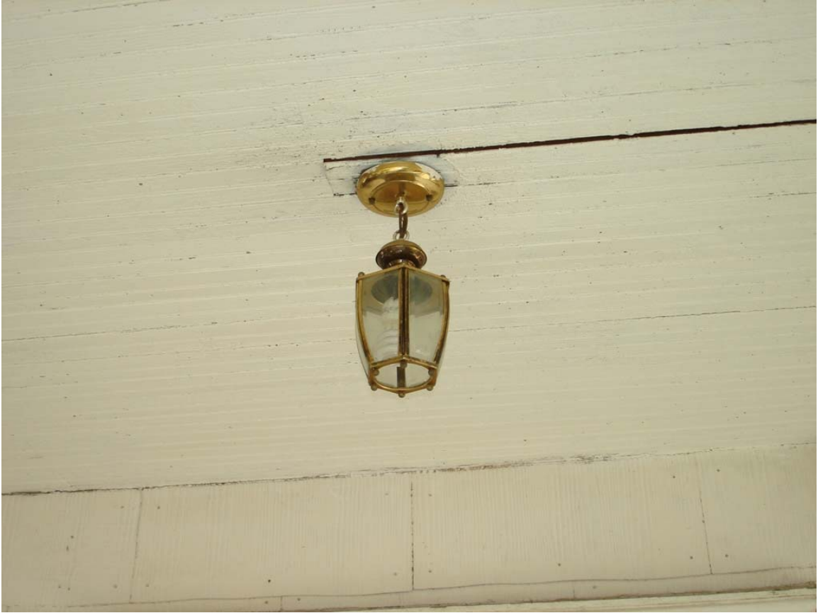
Request #8 – Existing porch ceiling light.
