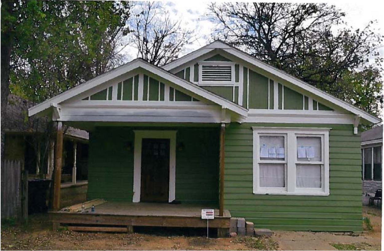
Front façade, after majority of exterior repair work and painting completed. Porch repair, including foundation, already started (with a routine maintenance CA).
