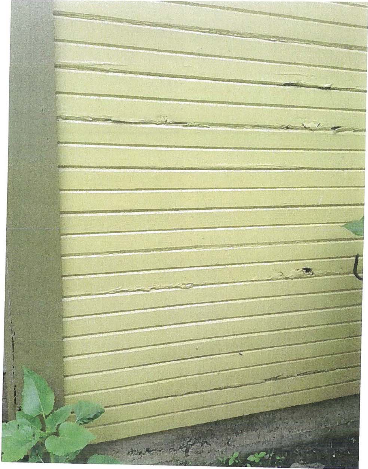
Rotten garage siding.
