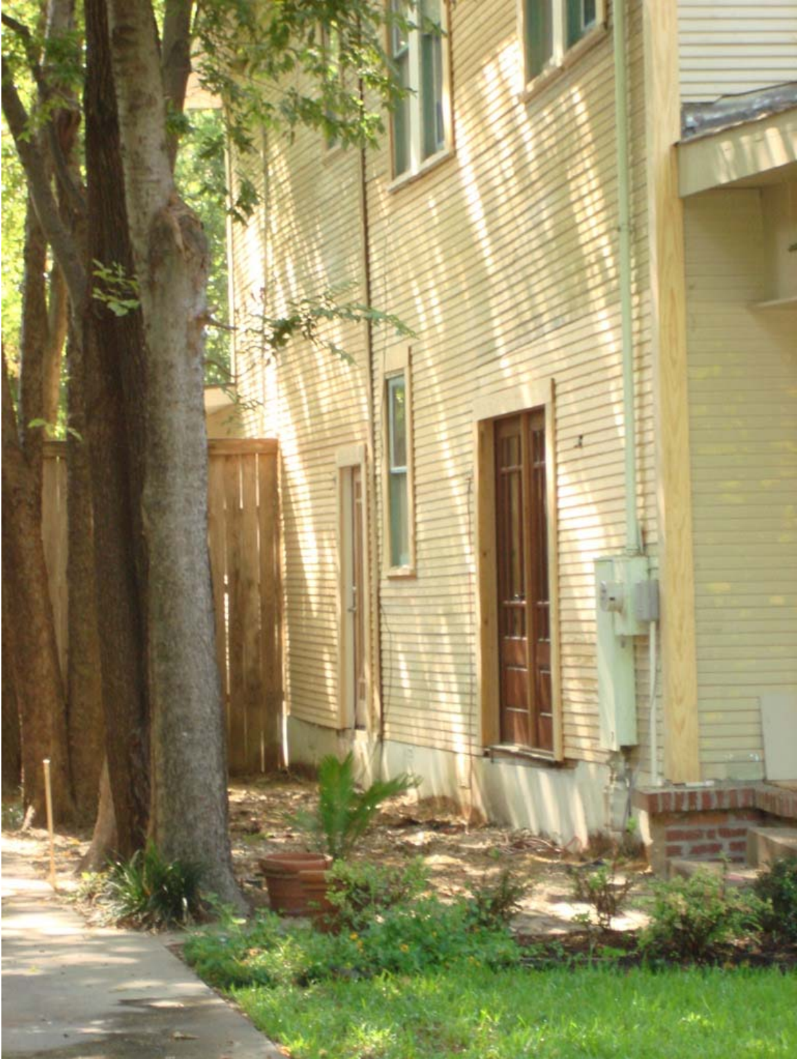
Partial east elevation showing location of side doors and two balconies that were removed.
