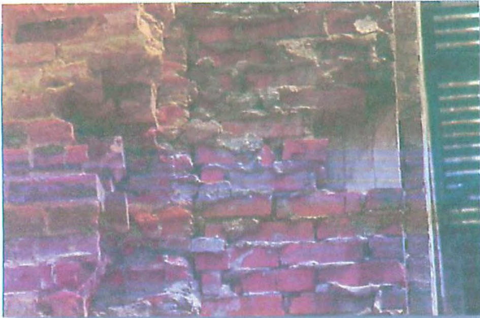
15. S.W. CORNER OF BUILDING, BROKEN MASONRY & LOOSE MORTAR
