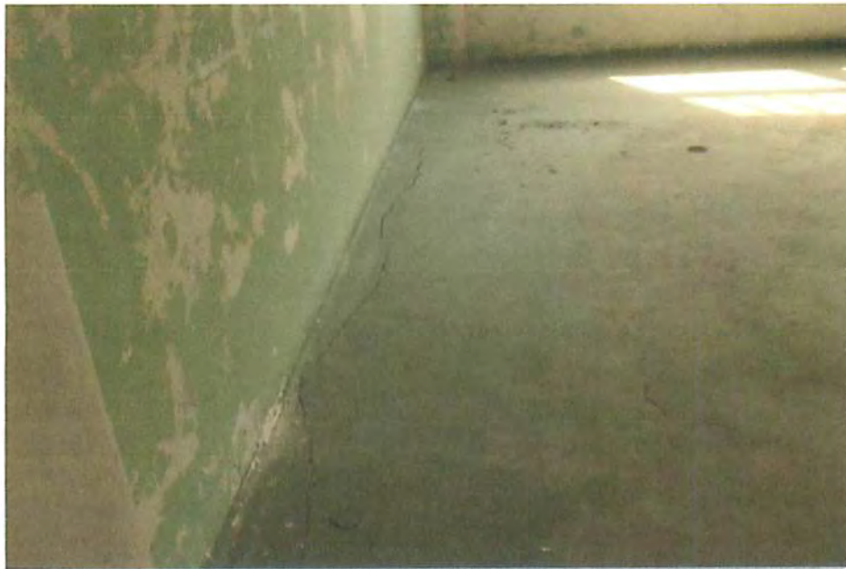
5. TYPICAL CRACKS, FLOORS 2-5.
