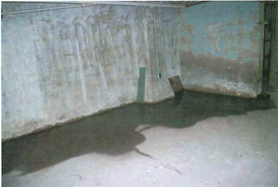
21. BASEMENT, WEST WALL WATER BUILD-UP.
