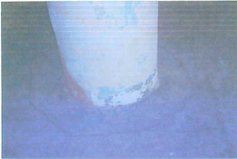
6. TYPICAL CRACKING AT COLUMNS, FLOORS 2-5.
