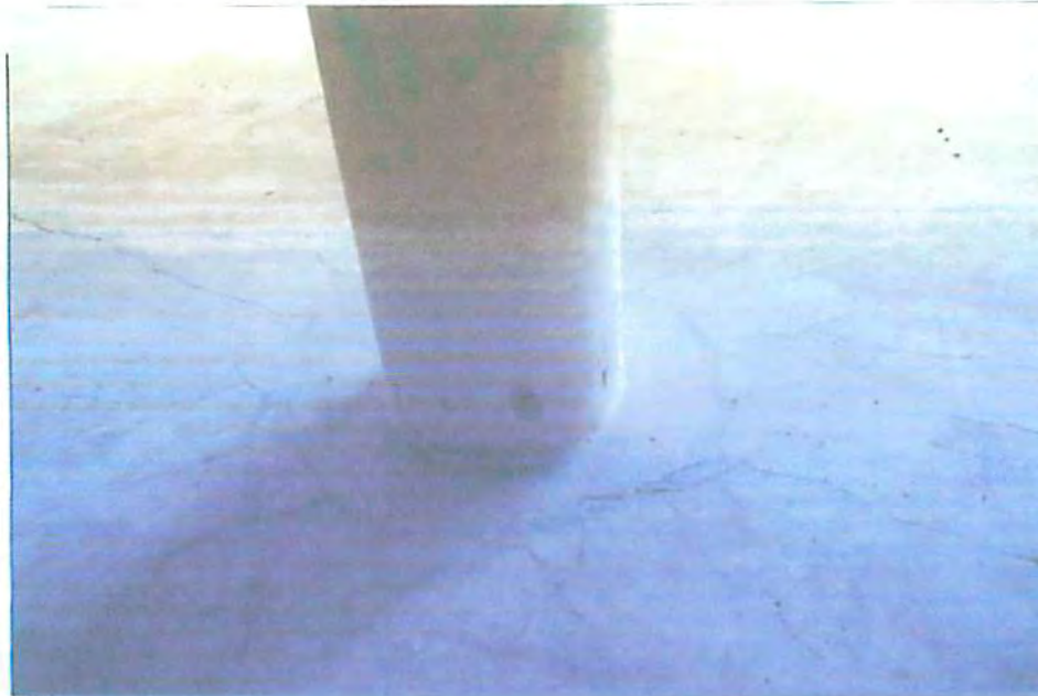
8. TYPICAL AT FLOORS 2,3,4,5 WITH MANY SLAB CRACKS
