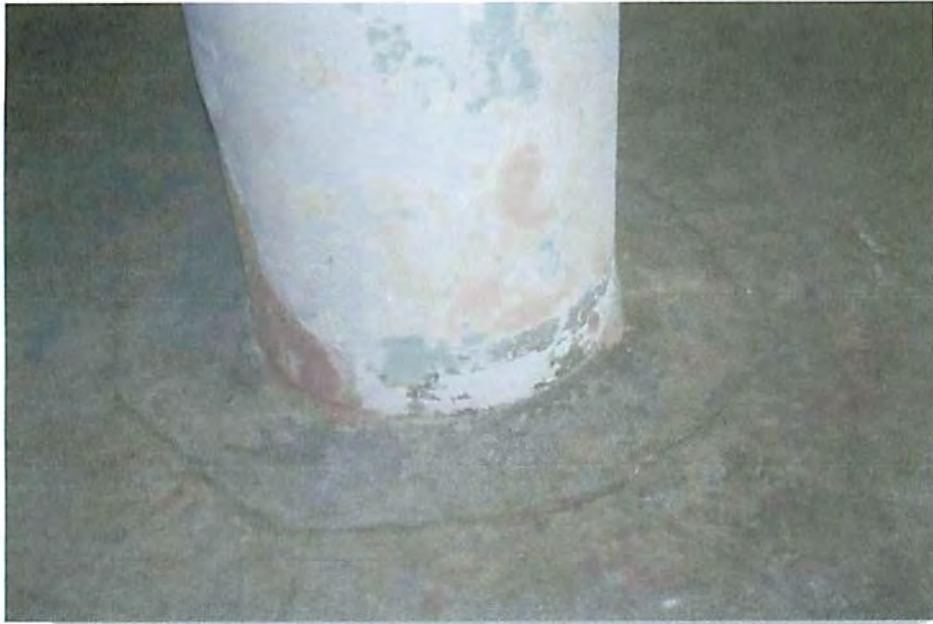
6. TYPICAL CRACKING AT COLUMNS, FLOORS 2-5.
