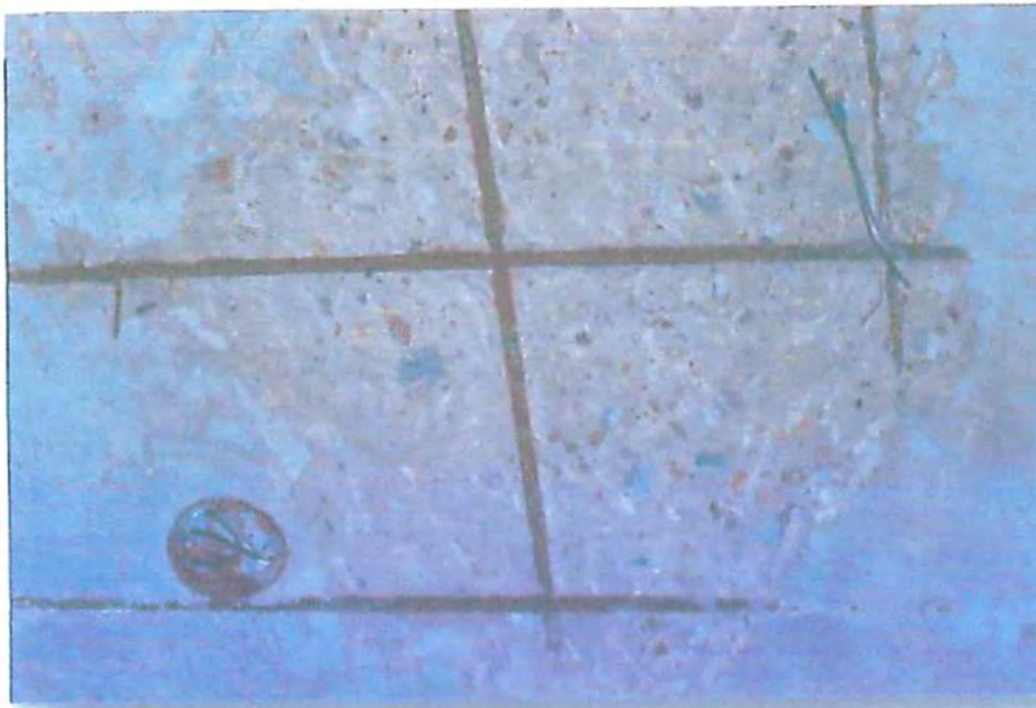
2. 2 ND FLOOR "FIRST FLOOR CEILING" TYPICAL. AND RUSTED REINFORCING
