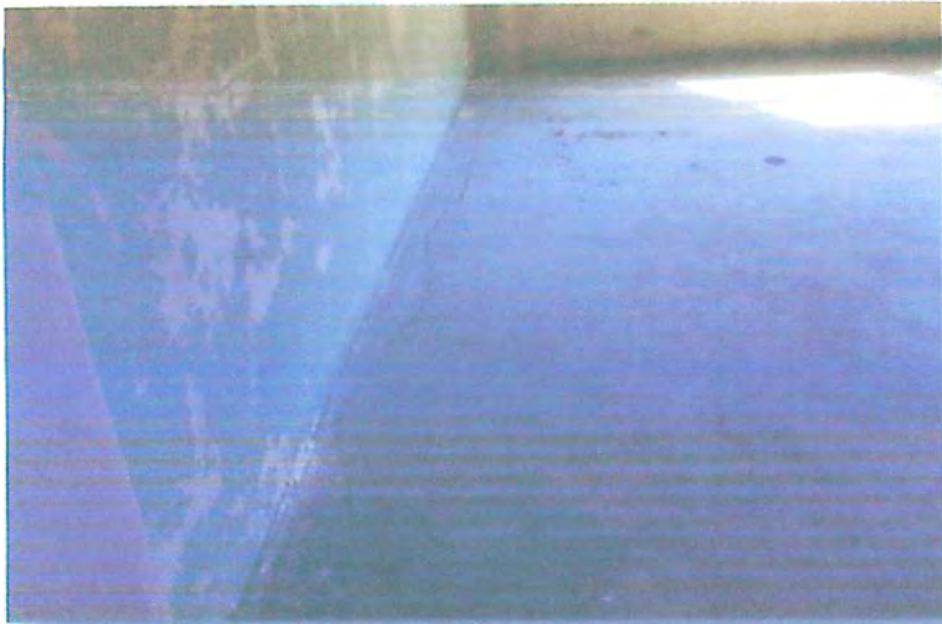
5. TYPICAL CRACKS, FLOORS 2-5.
