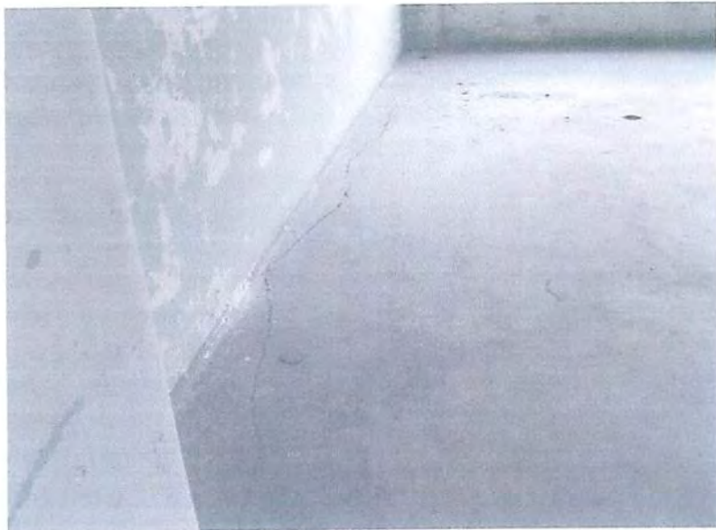
TYPICAL CRACK - LEVEL 2,3,4,5. - EAST, WEST, AND SOUTH SIDES -P5
