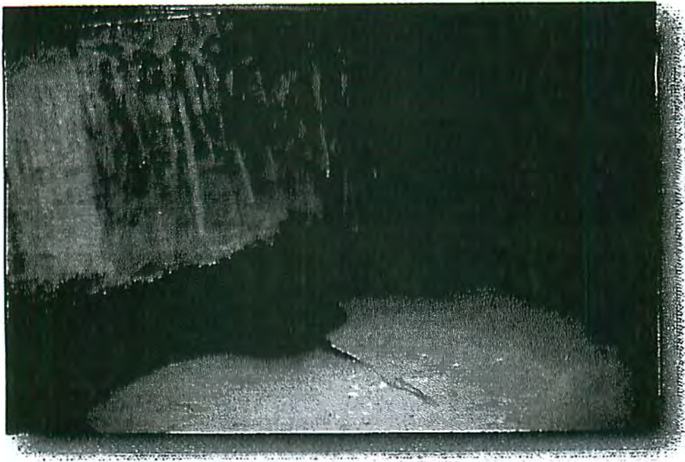
21. BASEMENT, WEST WALL WATER BUILD-UP.
