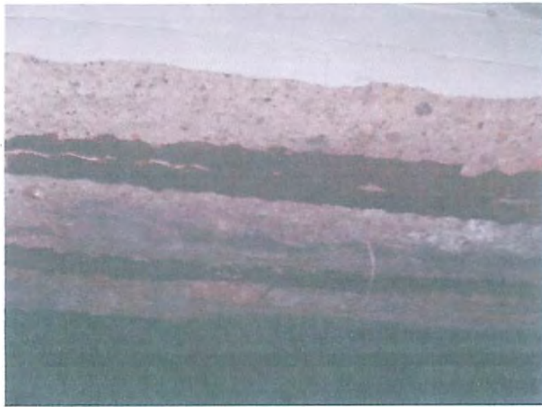
NO COVER FOR BOTTOM OF BEAM SUPPORT OF SIDEWALK – P12
