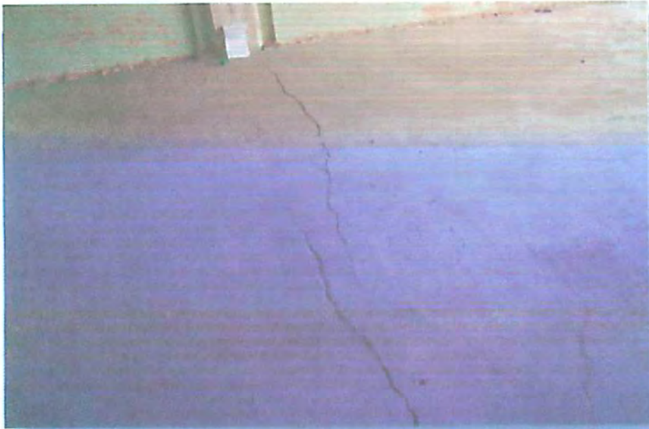
9. 3 RD FLOOR WITH TYPICAL LARGE CRACKS
